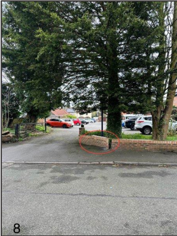
Picture 9. T8-Monterey cypress with low branches over path. Stem growth is damaging wall as shown by red circle.
