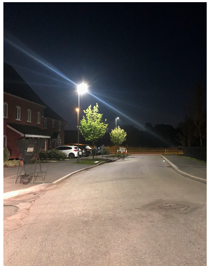
Figure B36 Luminaire, Southcroft Drive
