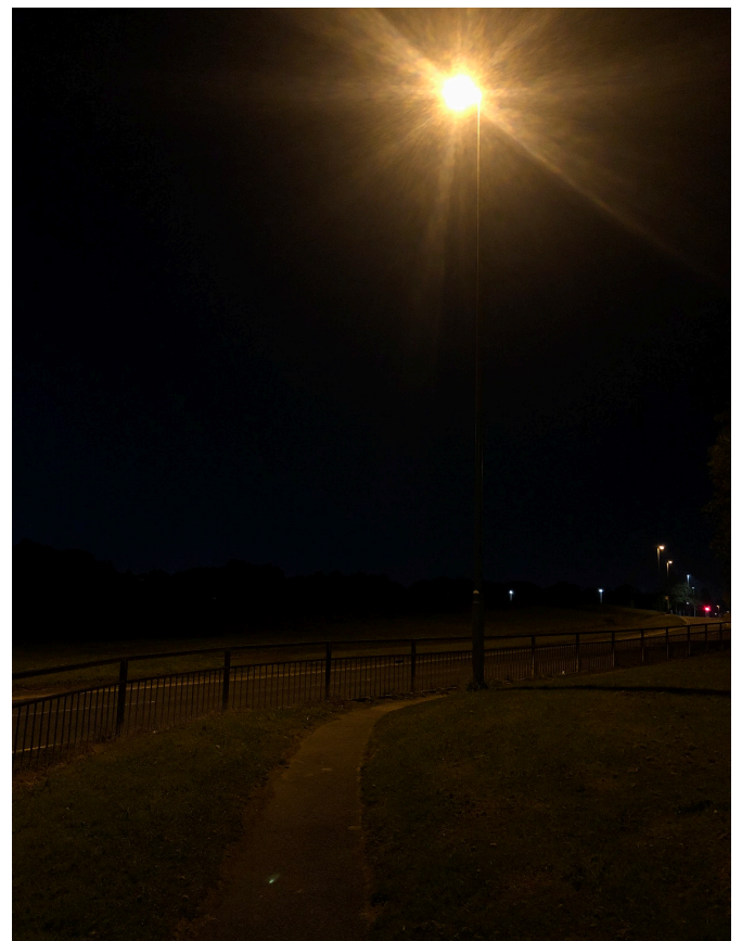
Figure B32 Luminaire, Fallowfield/Headbolt Ln.
