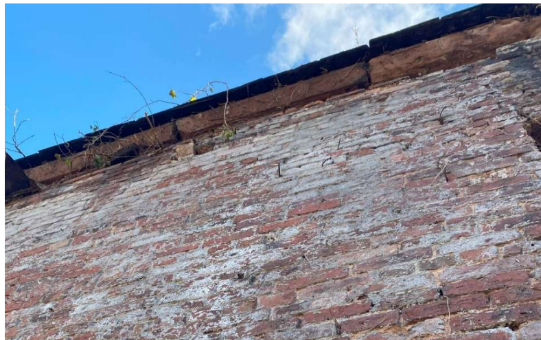
Plate 8 – Red stone blocks to be re-bed to the northwest rear elevation.
