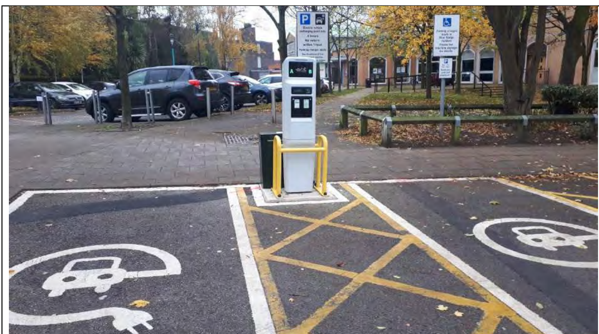
Photo 43 – Electric car charging station located on site
