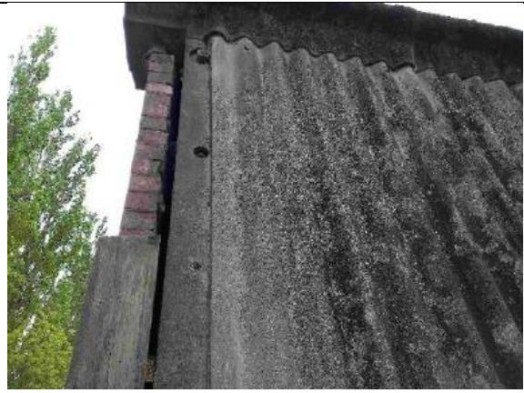
Photograph 14: Gaps present between adjoining walls on north-eastern corner of B2
