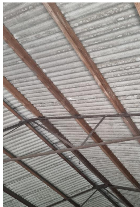
(Holes in the roof – Rusty stanchions)
