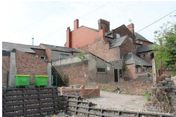
9. View showing site level changes and site walls requiring remedial.
