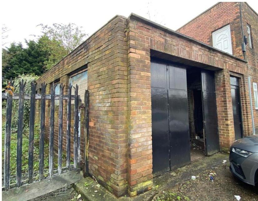
Structurally Unsound Rear Boundary Wall
