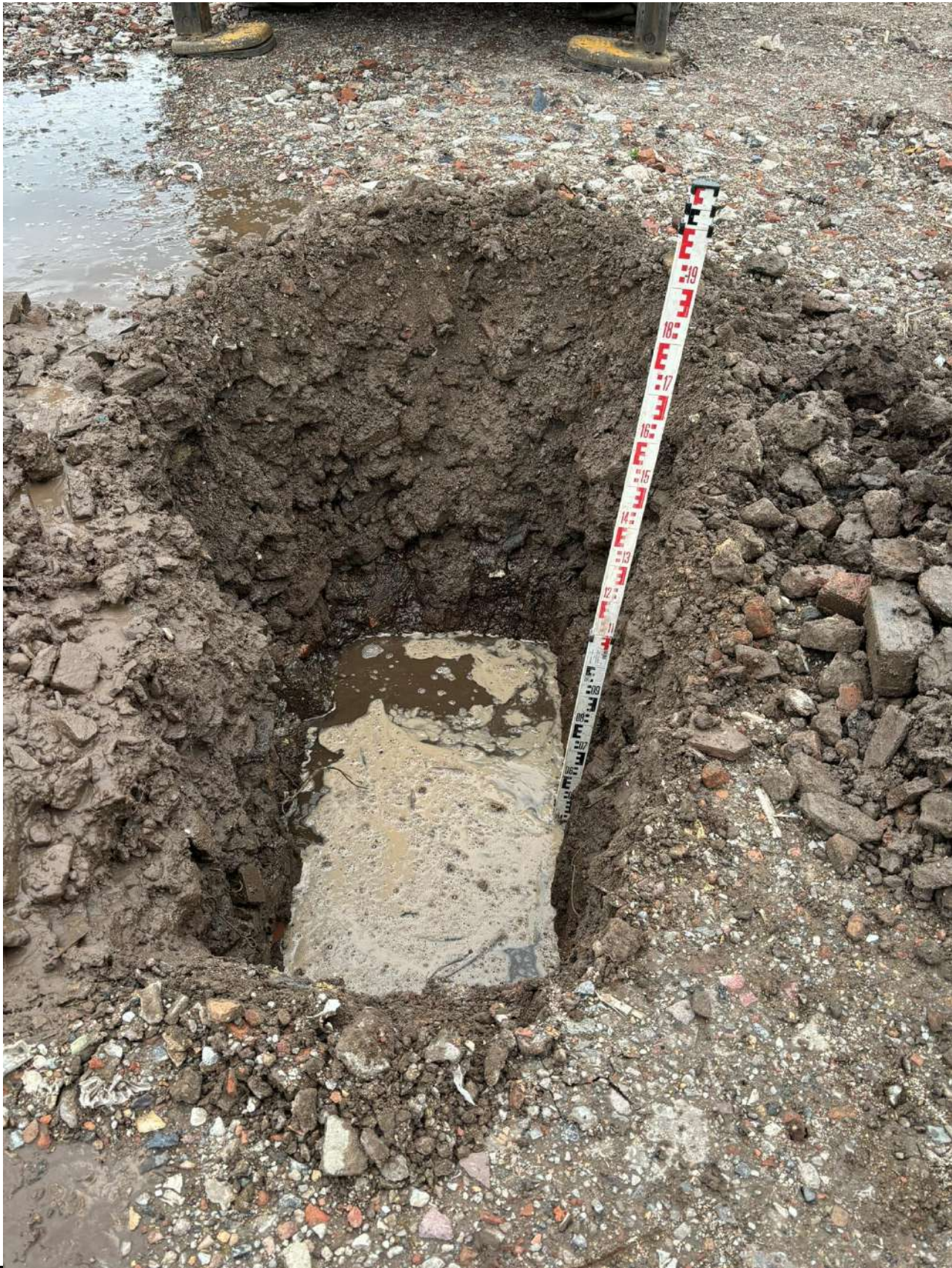
Plate 14: TP13 showing the ingress of water and depth of the excavation
