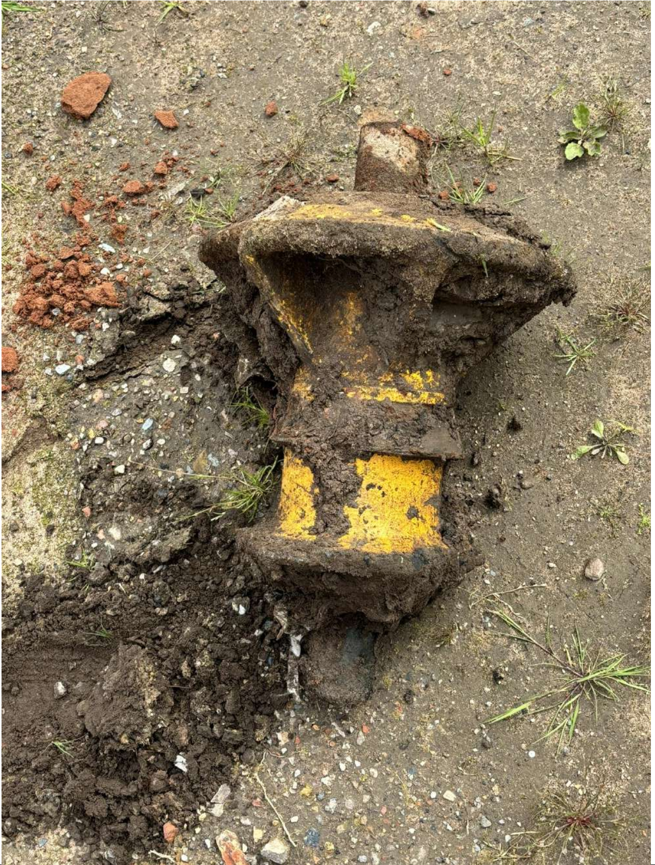
Plate 13: TP12 obstruction found during the excavation
