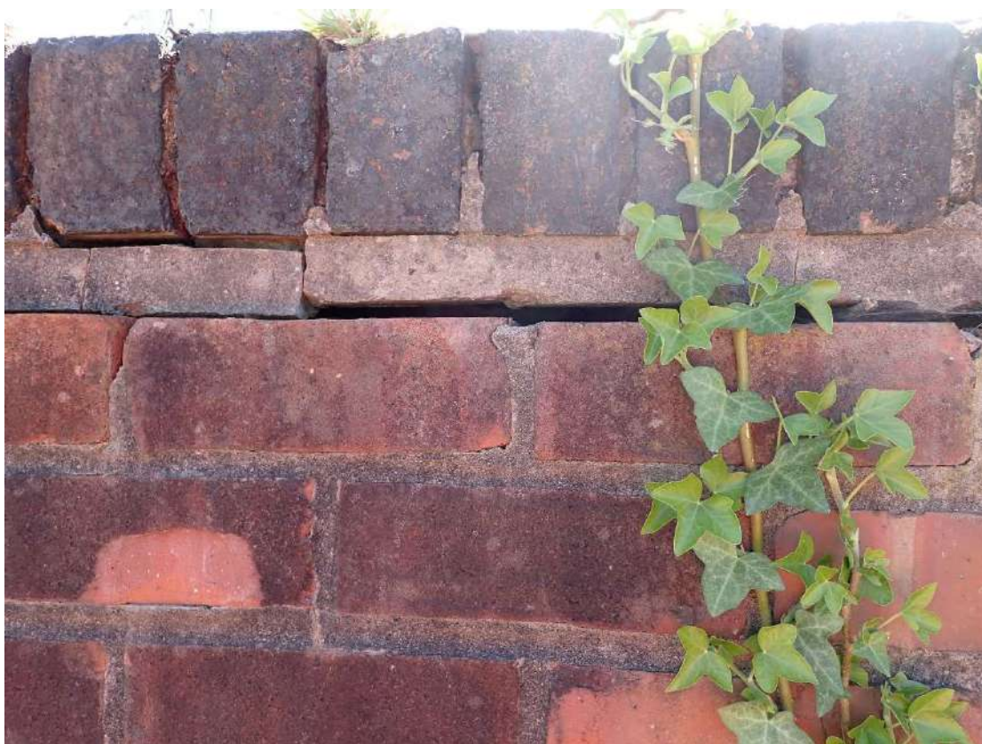
Photograph 14. Example of a cavity within the mortar of the redbrick wall.
