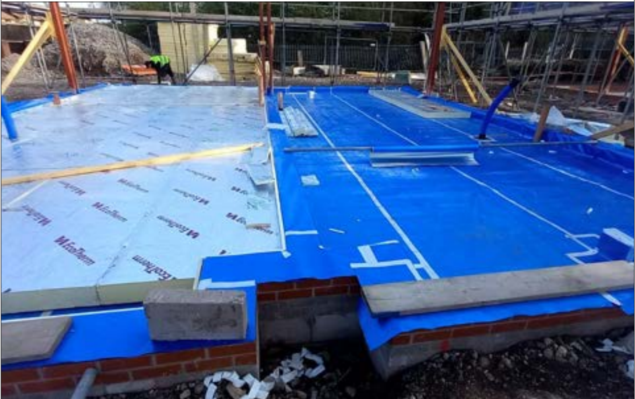
Plate 1: Plots 1 & 2 gas membrane general condition.
