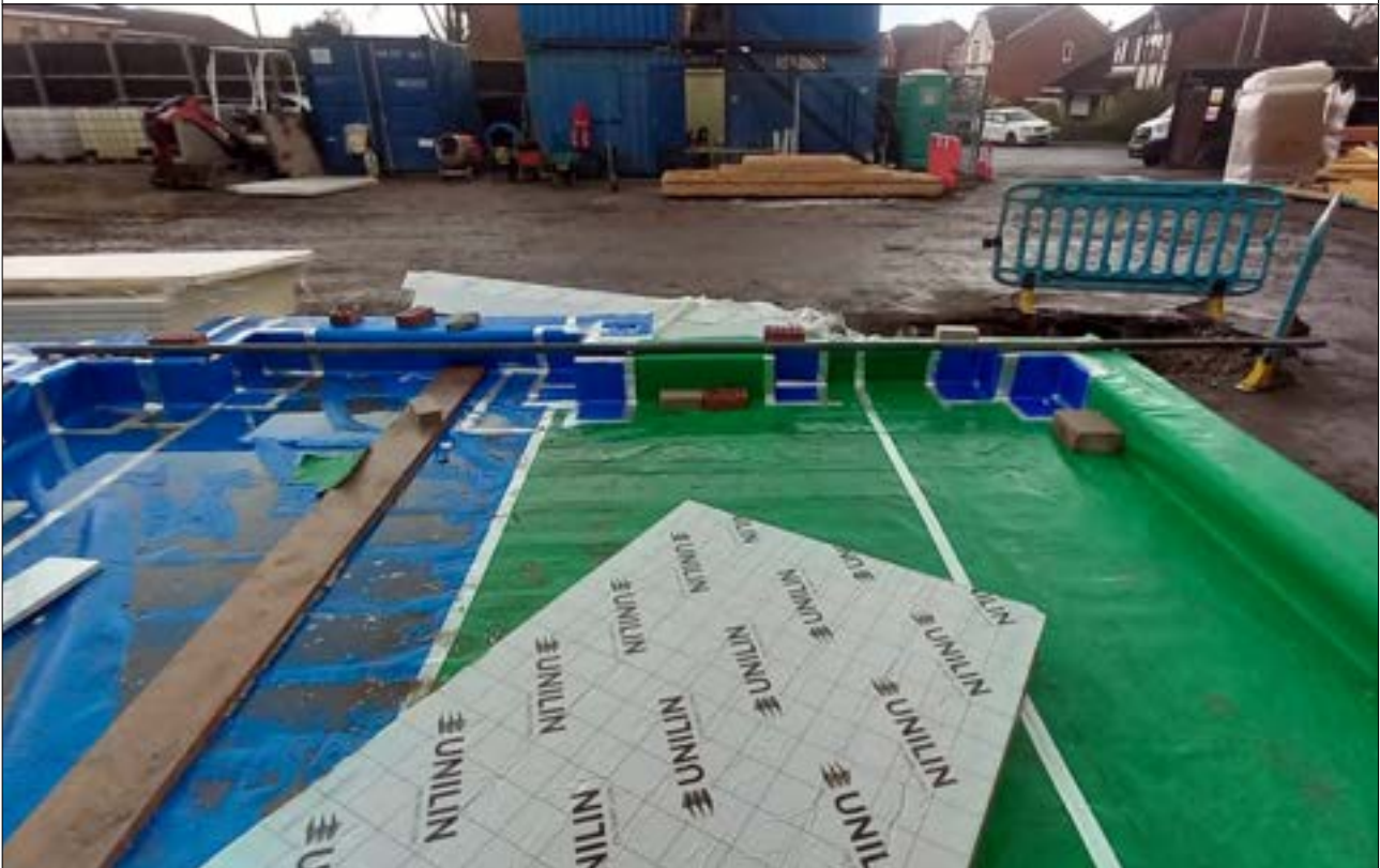
Plate 17: Plots 5, 6 & 7 gas membrane general condition.
