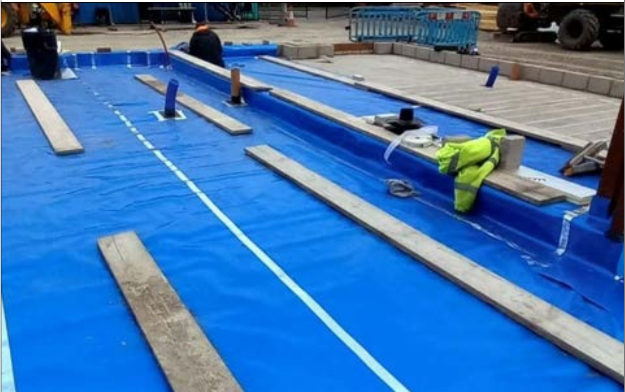
Plate 18: Plots 5, 6 & 7 gas membrane general condition.
