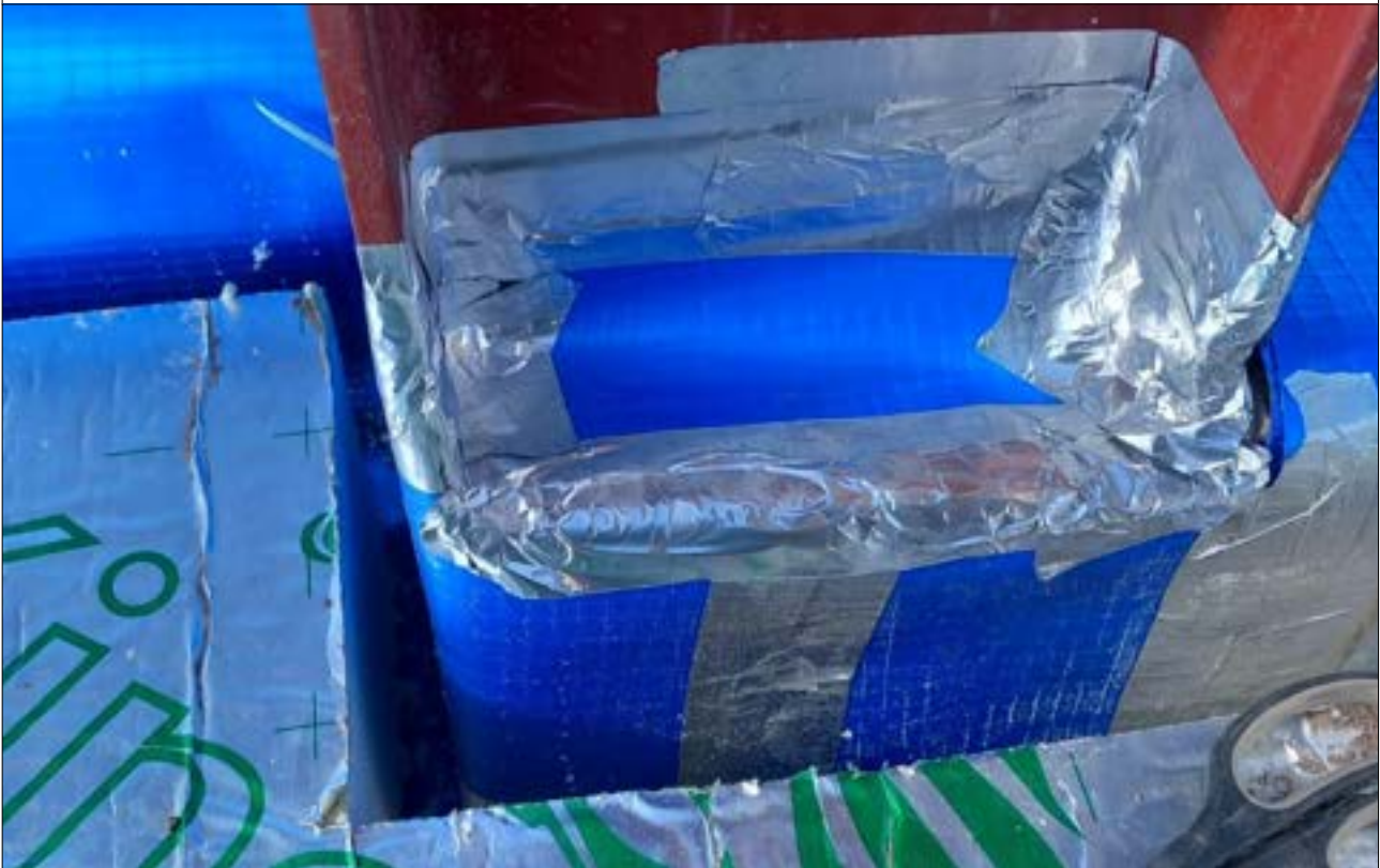
Plate 11: Plots 3 & 4 gas membrane general condition.
