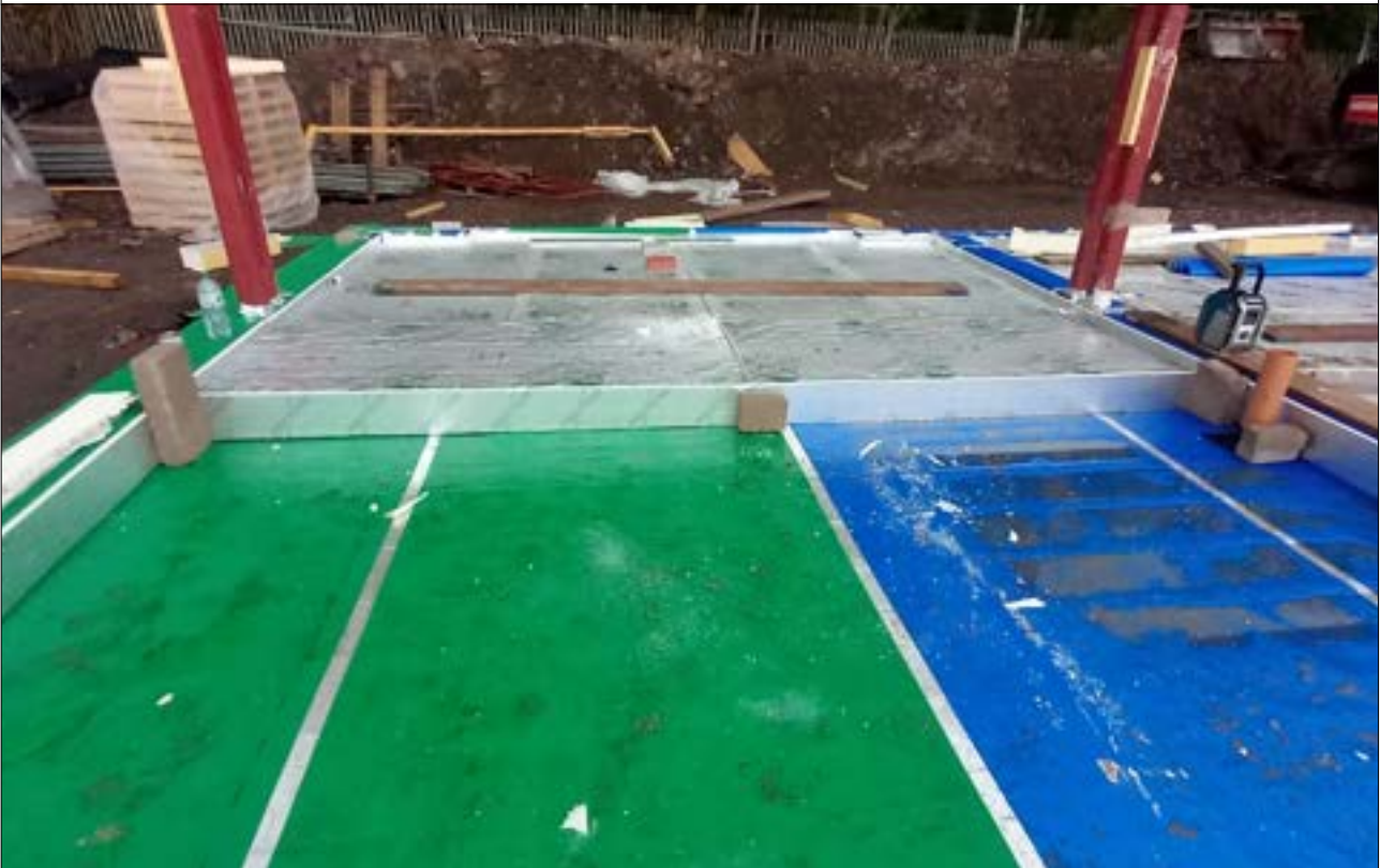
Plate 19: Plots 5, 6 & 7 gas membrane general condition.
