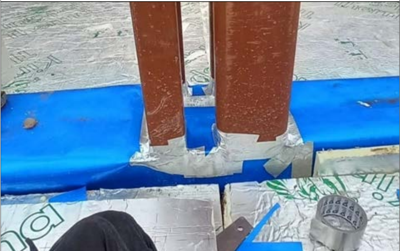
Plate 16: Plots 3 & 4 gas membrane general condition.
