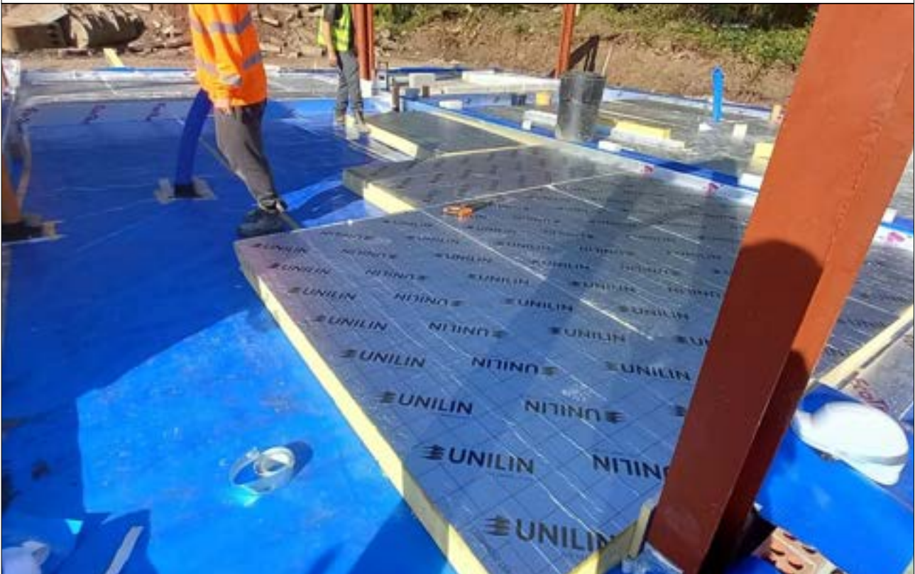
Plate 28: Plots 8 & 9 gas membrane general condition.
