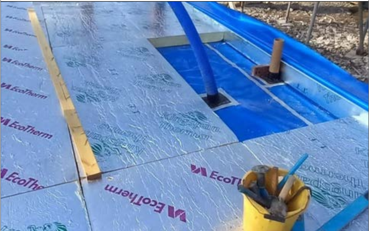
Plate 6: Plots 1 & 2 gas membrane general condition.
