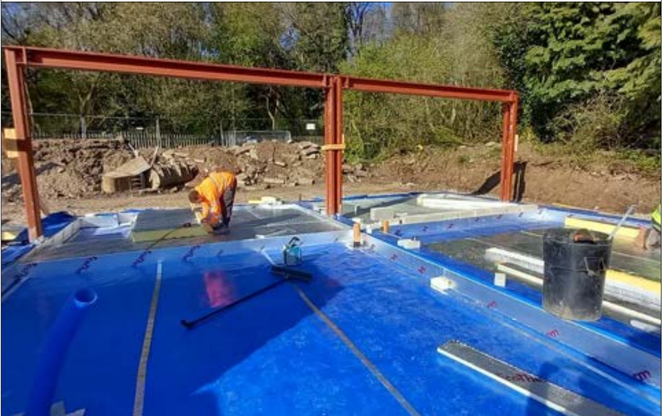
Plate 25: Plots 8 & 9 gas membrane general condition.
