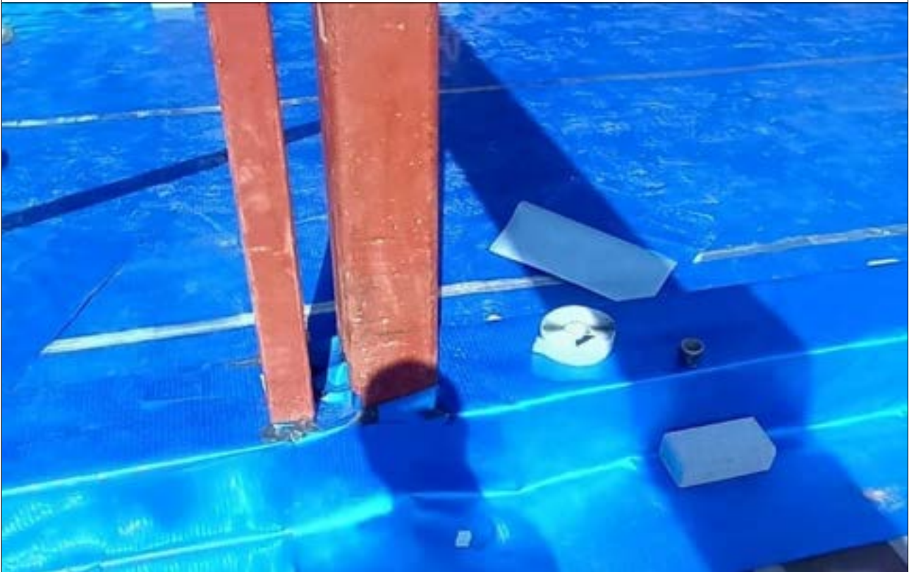
Plate 31: Plots 8 & 9 gas membrane general condition.
