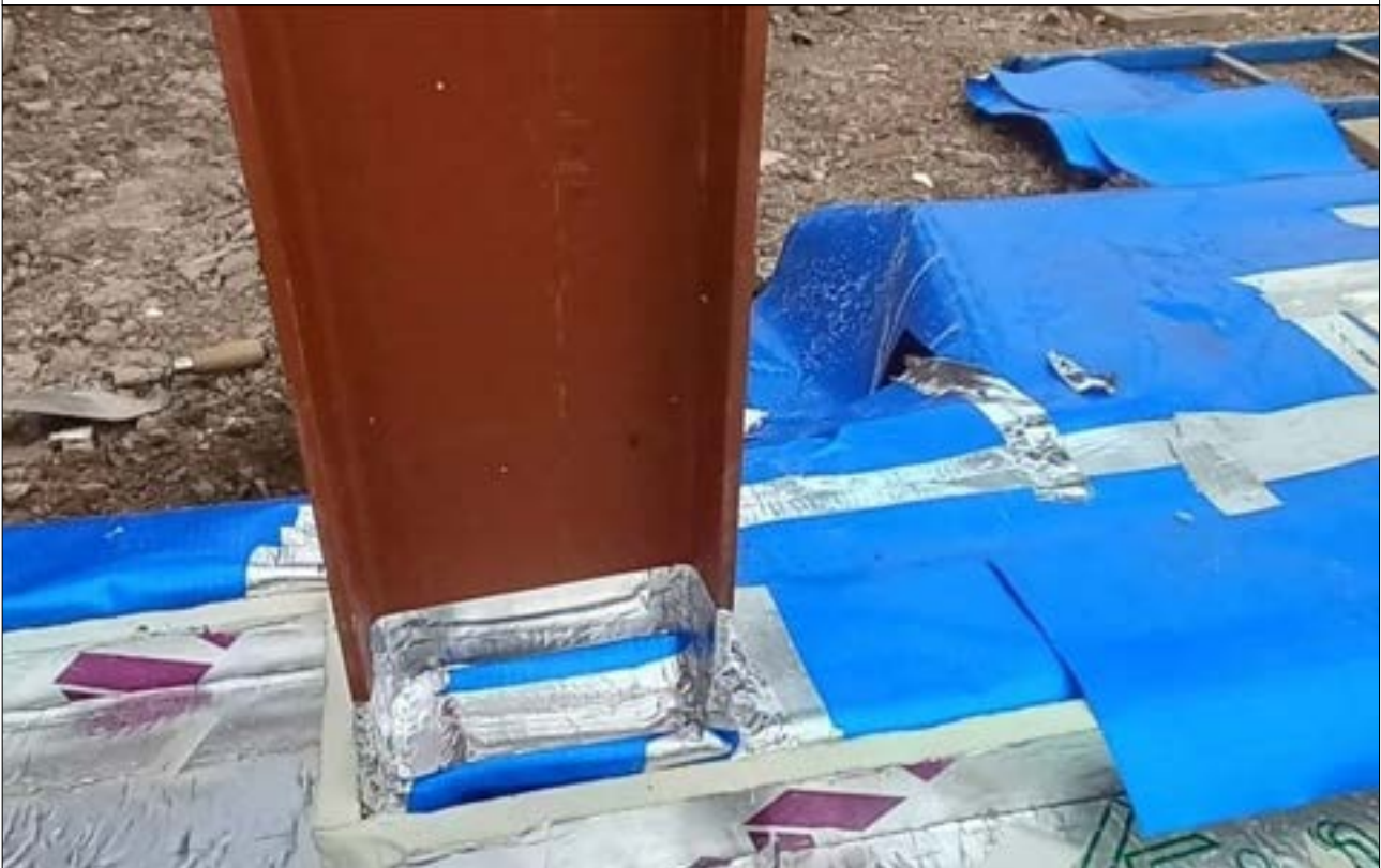
Plate 12: Plots 3 & 4 gas membrane general condition.
