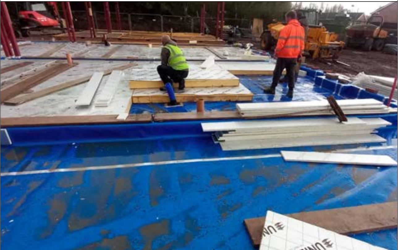
Plate 20: Plots 5, 6 & 7 gas membrane general condition.
