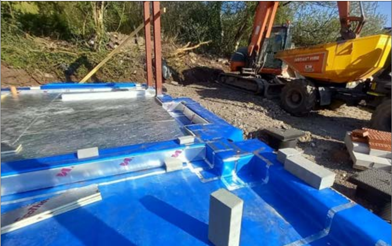
Plate 27: Plots 8 & 9 gas membrane general condition.
