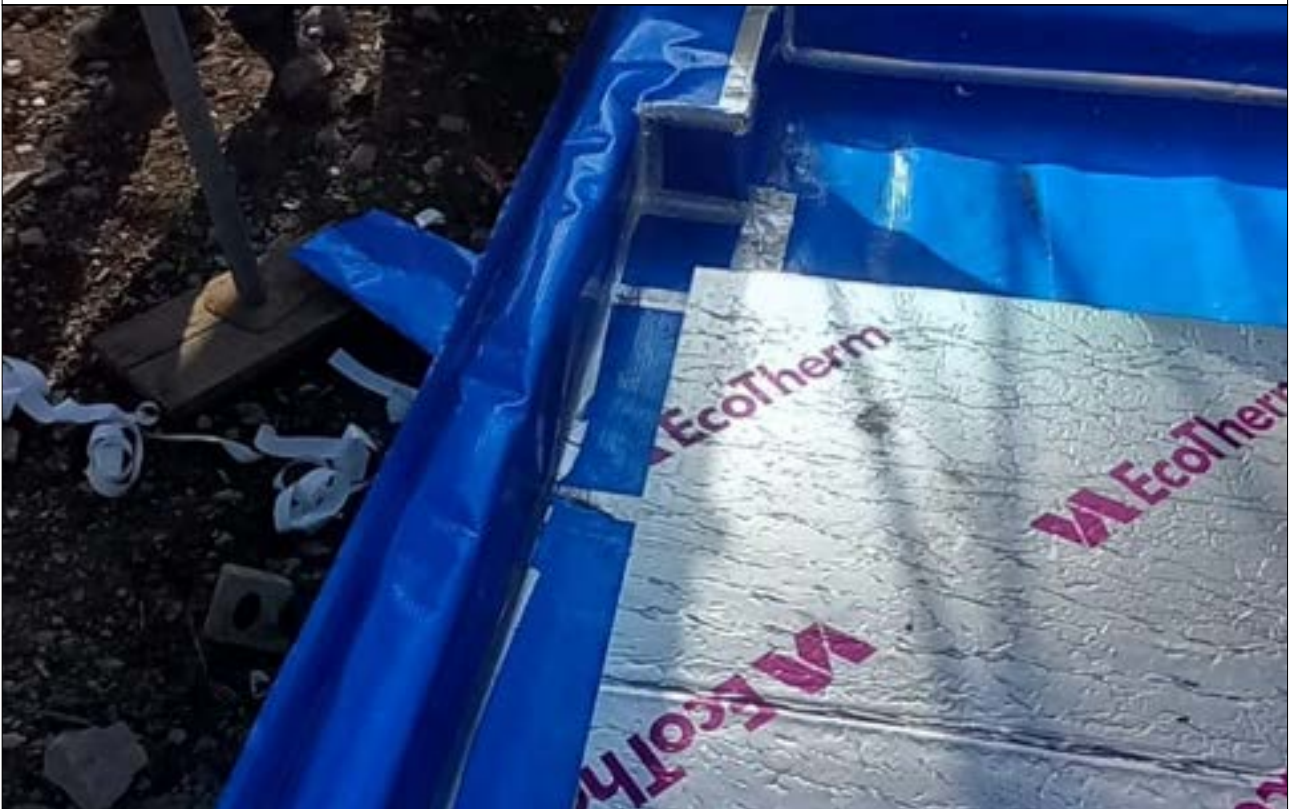
Plate 8: Plots 1 & 2 gas membrane general condition.
