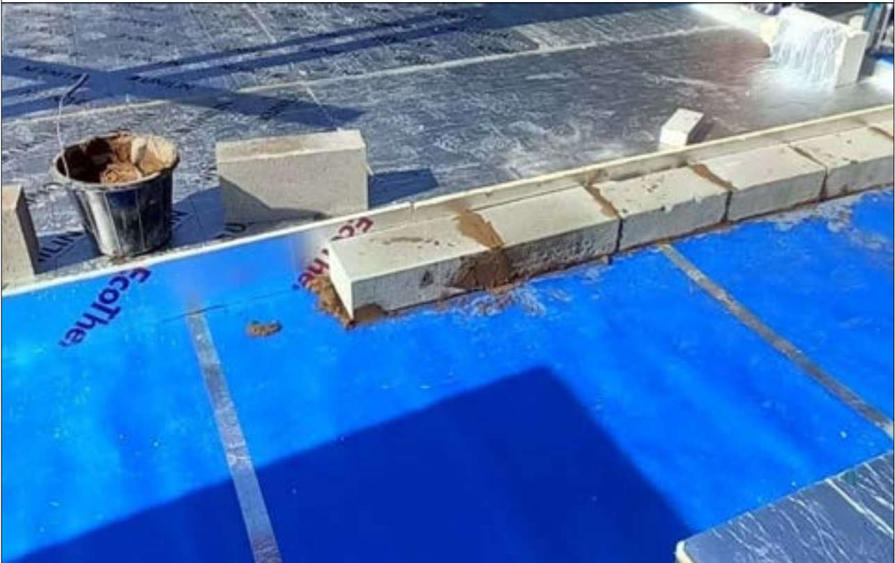
Plate 29: Plots 8 & 9 gas membrane general condition.
