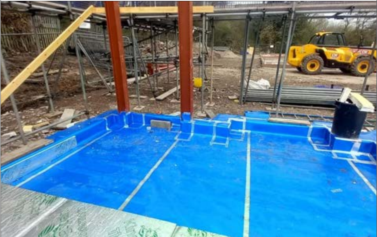
Plate 9: Plots 3 & 4 gas membrane general condition.
