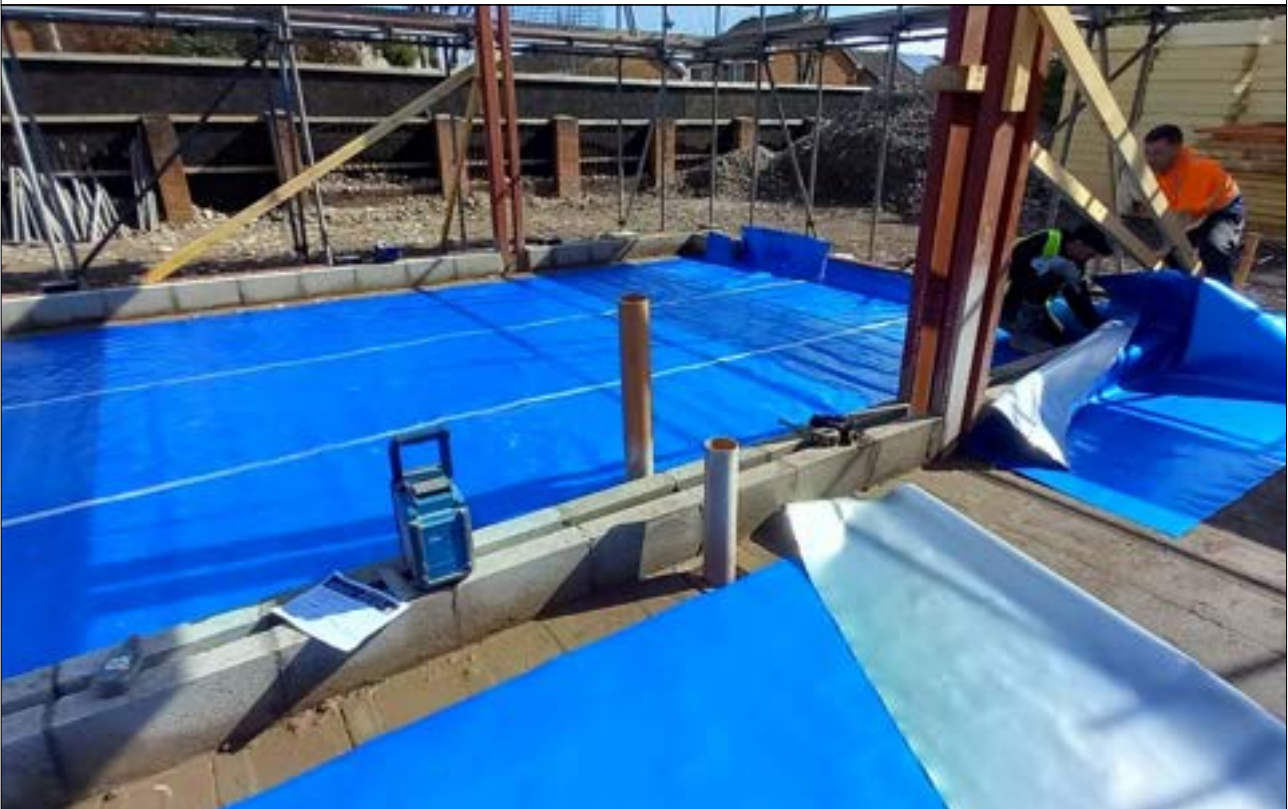
Plate 4: Plots 1 & 2 gas membrane general condition.
