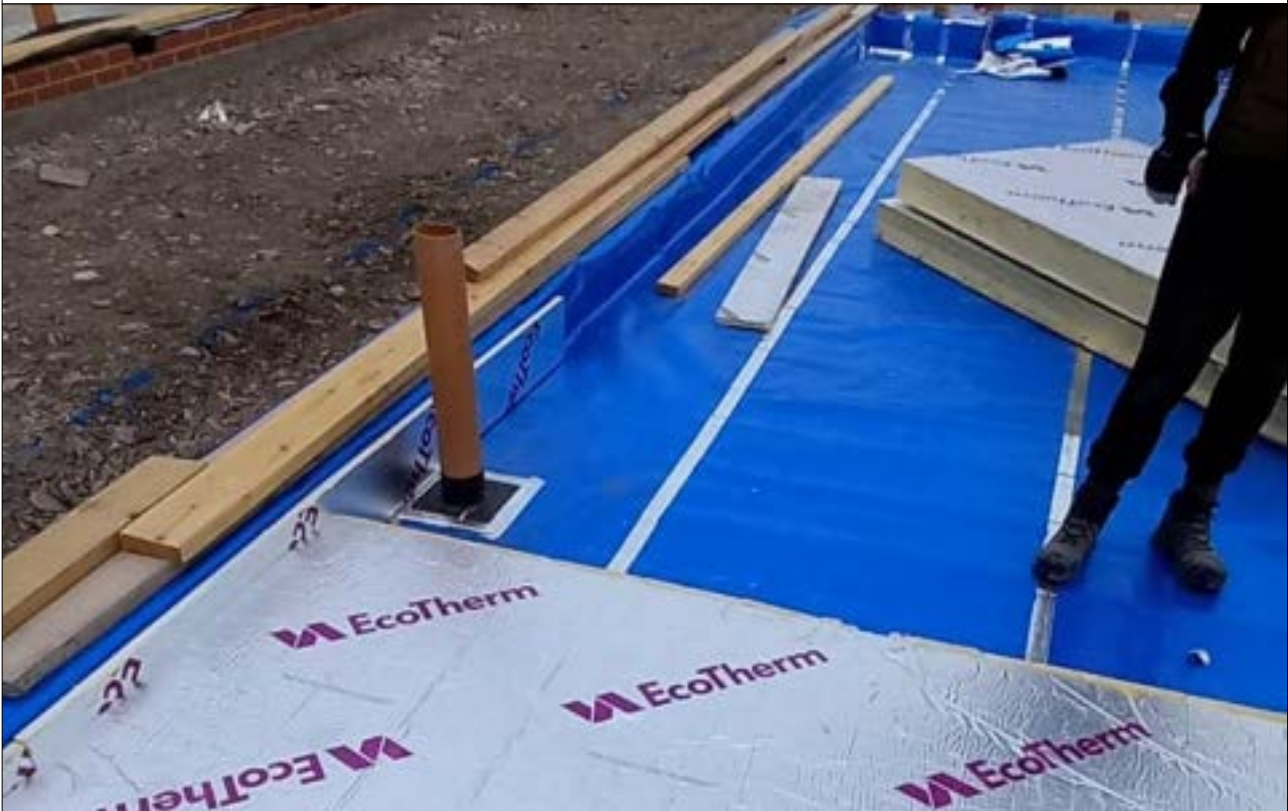
Plate 21: Plots 5, 6 & 7 gas membrane general condition.
