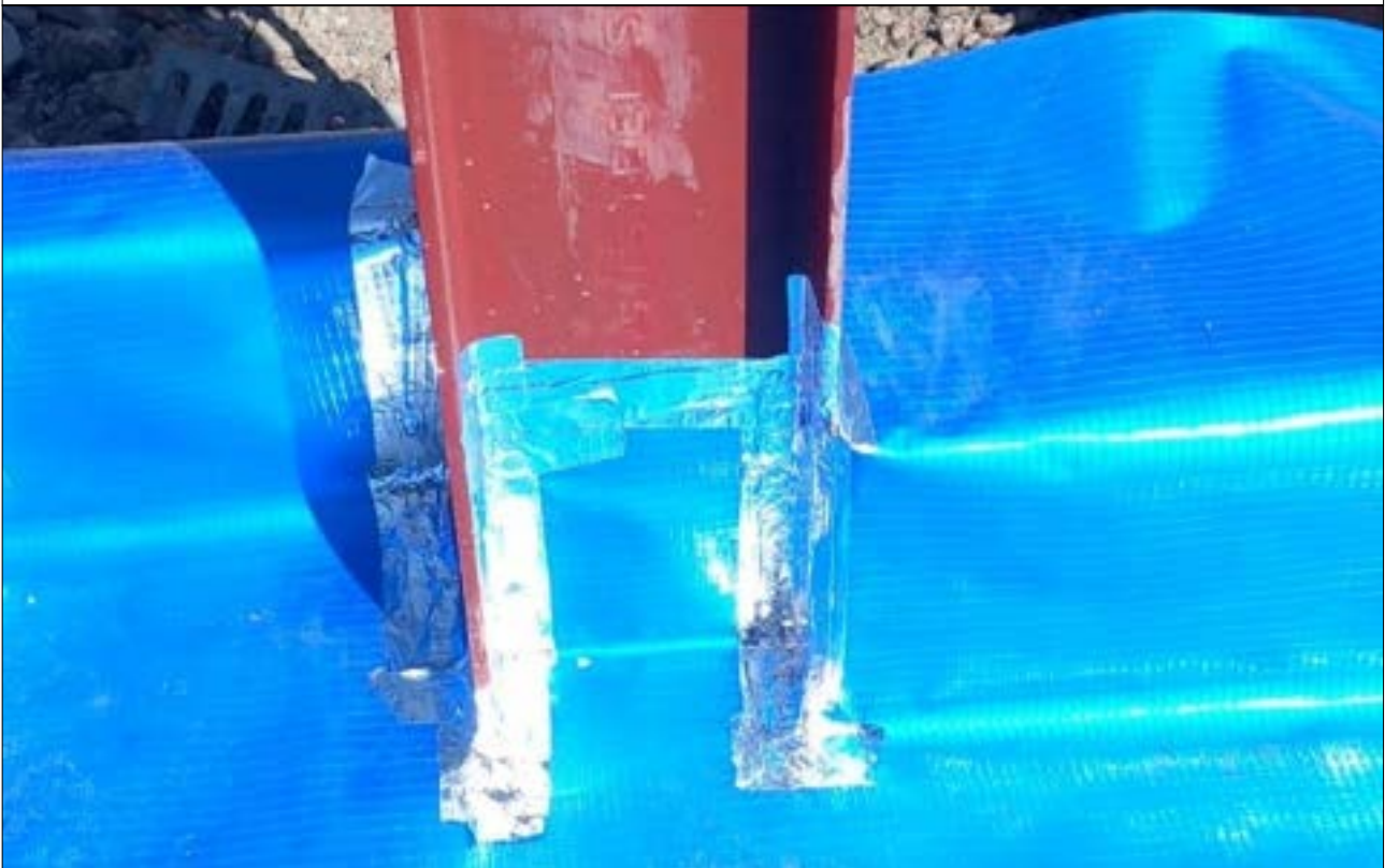
Plate 32: Plots 8 & 9 gas membrane general condition.
