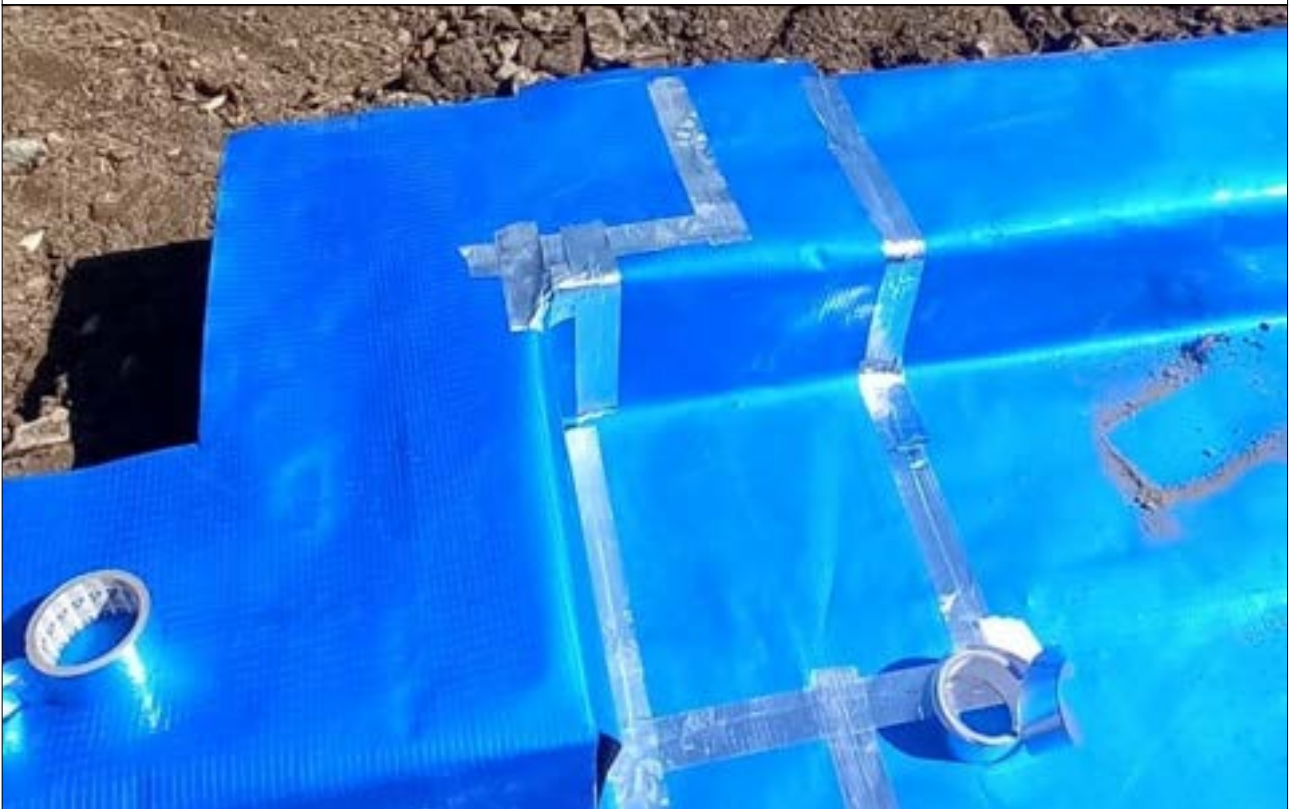
Plate 30: Plots 8 & 9 gas membrane general condition.
