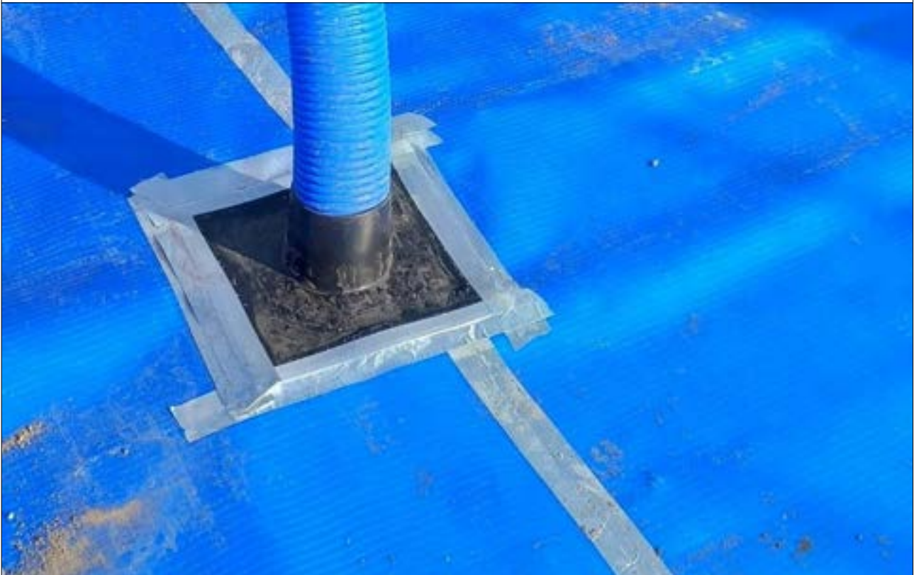
Plate 5: Plots 1 & 2 gas membrane general condition.
