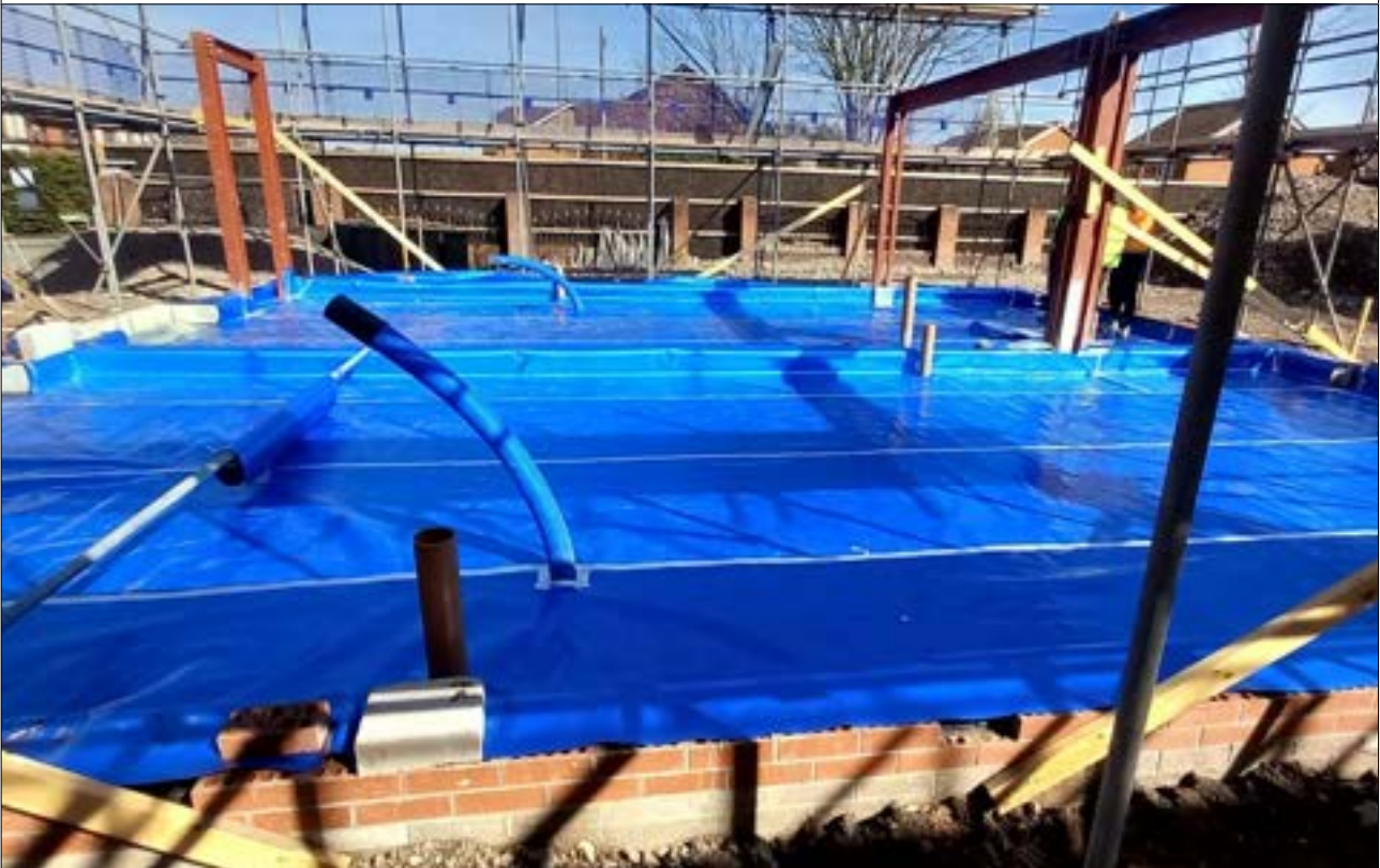
Plate 3: Plots 1 & 2 gas membrane general condition.
