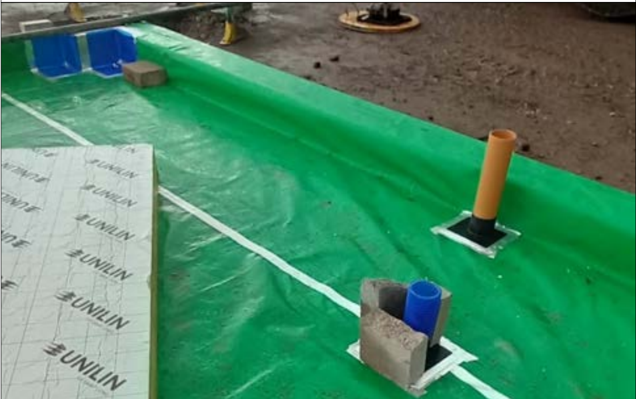
Plate 22: Plots 5, 6 & 7 gas membrane general condition.
