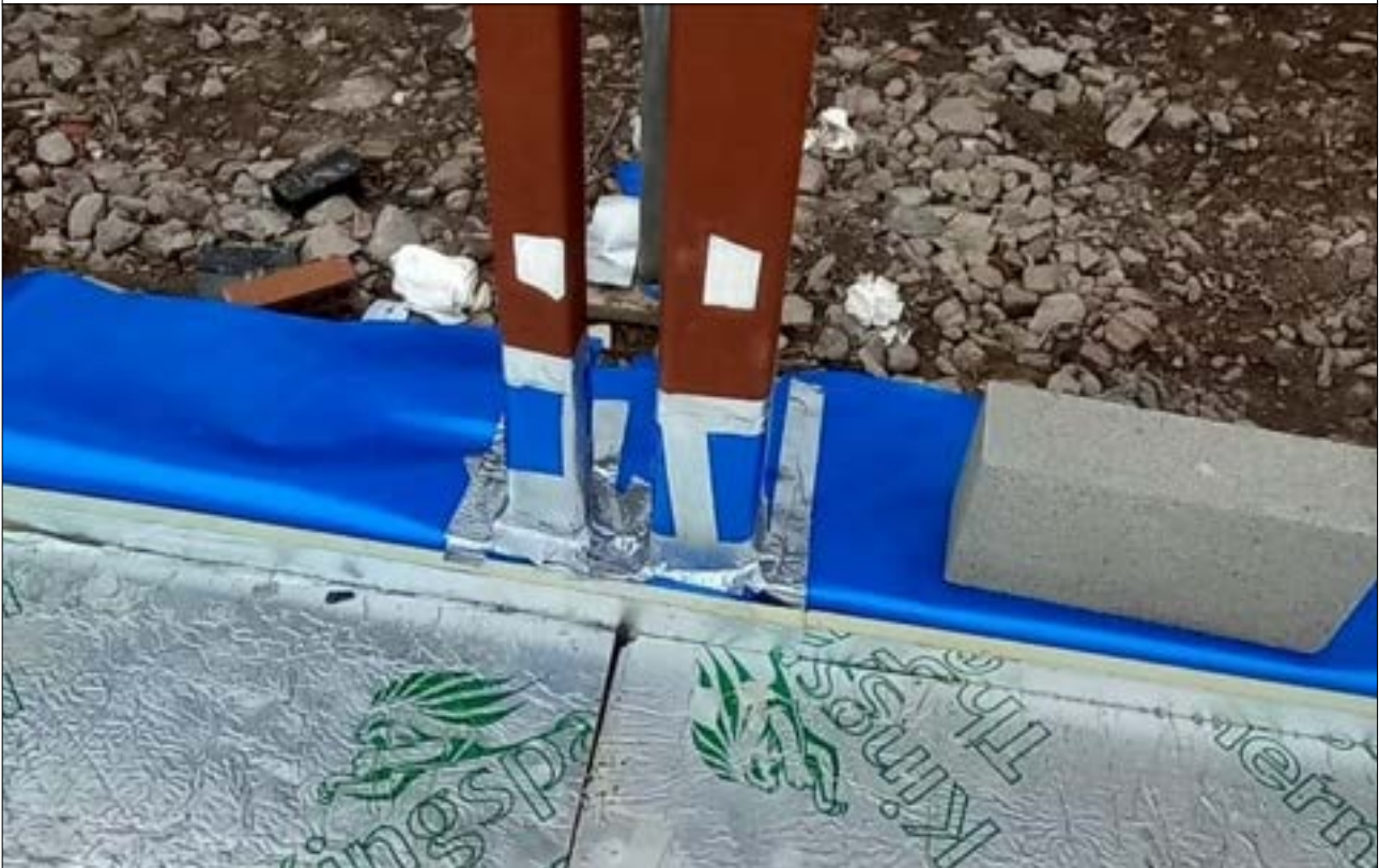
Plate 15: Plots 3 & 4 gas membrane general condition.
