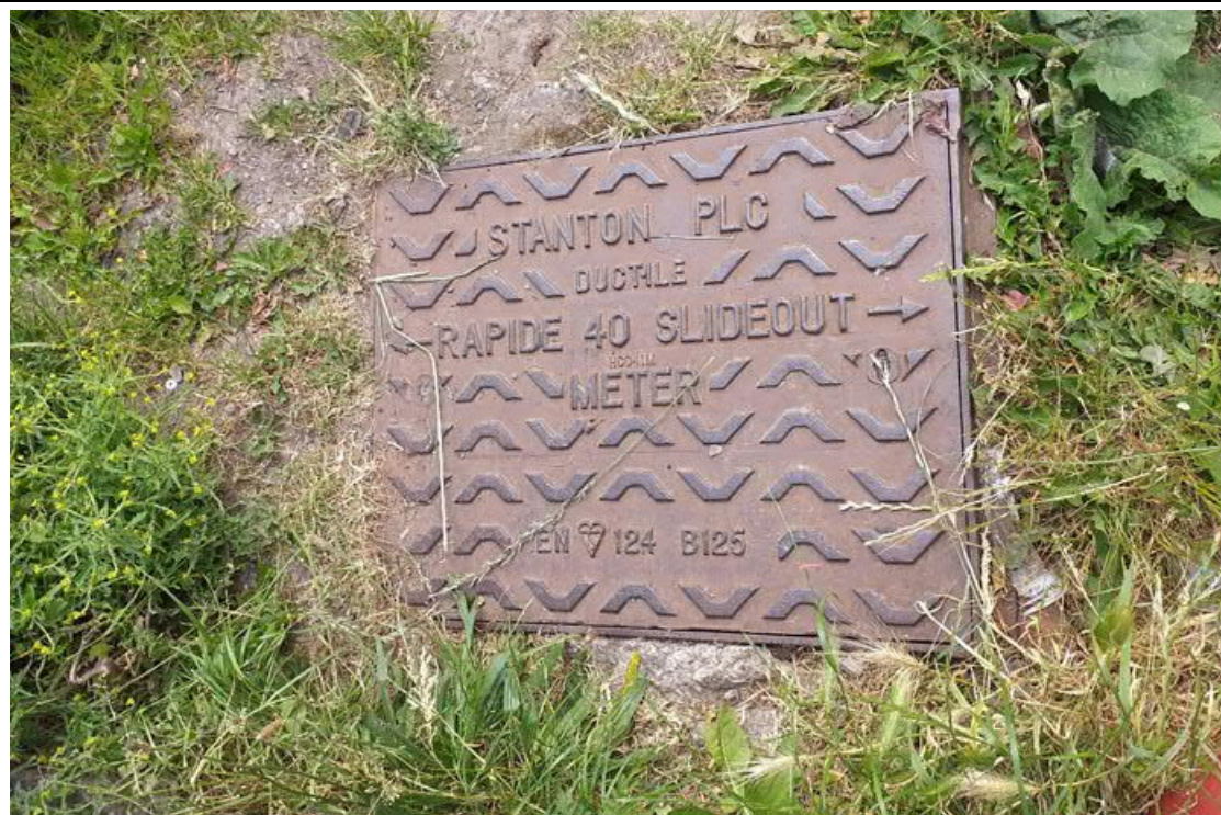
Photo 6: Stanton Plc ductile iron manhole cover adjacent to the gated vehicle access point from Windy Arbor Road.
