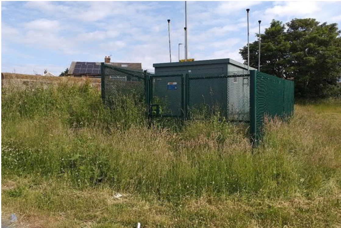
Photo 5: Onsite gas governor (potentially a pressure reduction station) owned by Cadent Gas according to signage. Station is secured by metal fencing and locked gate (photograph taken facing northwest).
