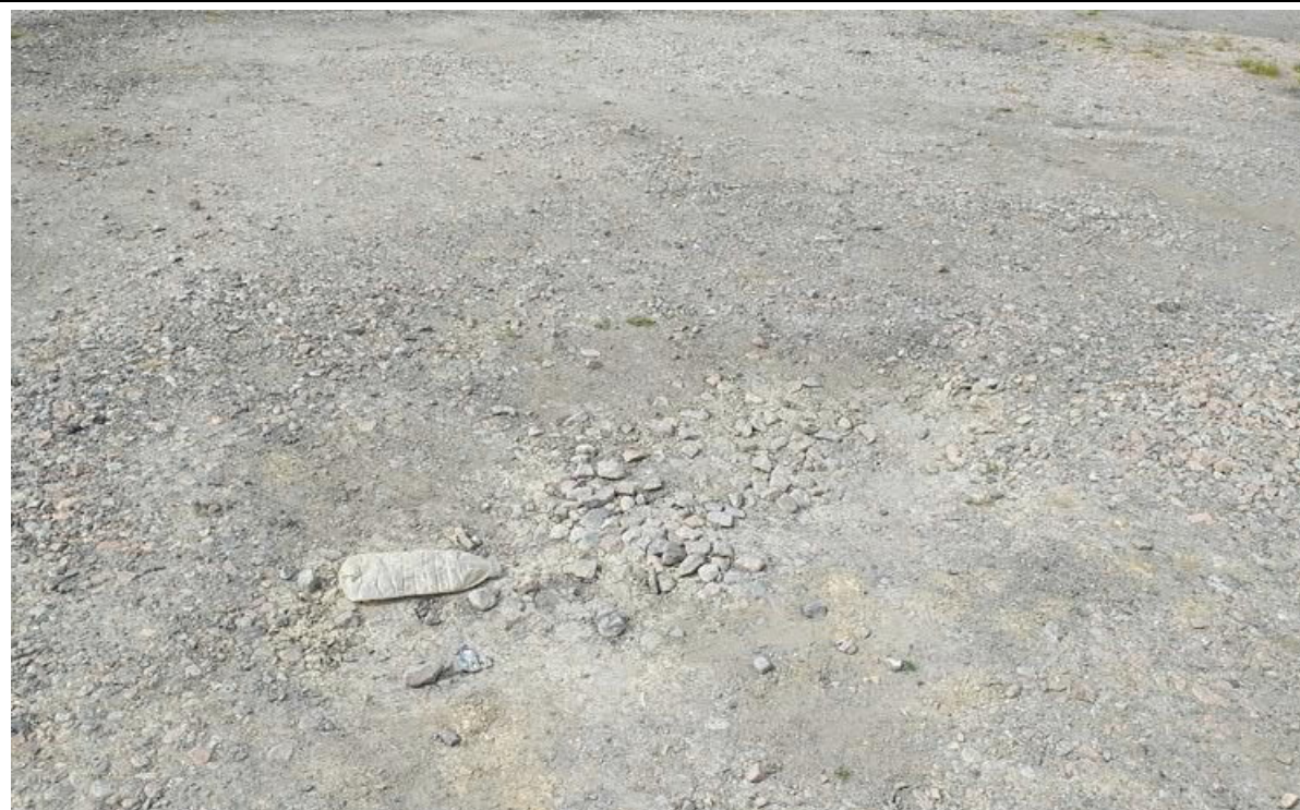
Photo 10: Car park surface composed of fine to coarse gravel of granite and limestone. Surface is uneven and is in poor condition.
