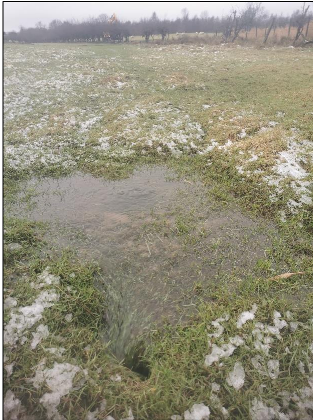
Photo 11: View north west in the central site section showing water uprising and sinking into a hole. This may be a collapsed land drain.
