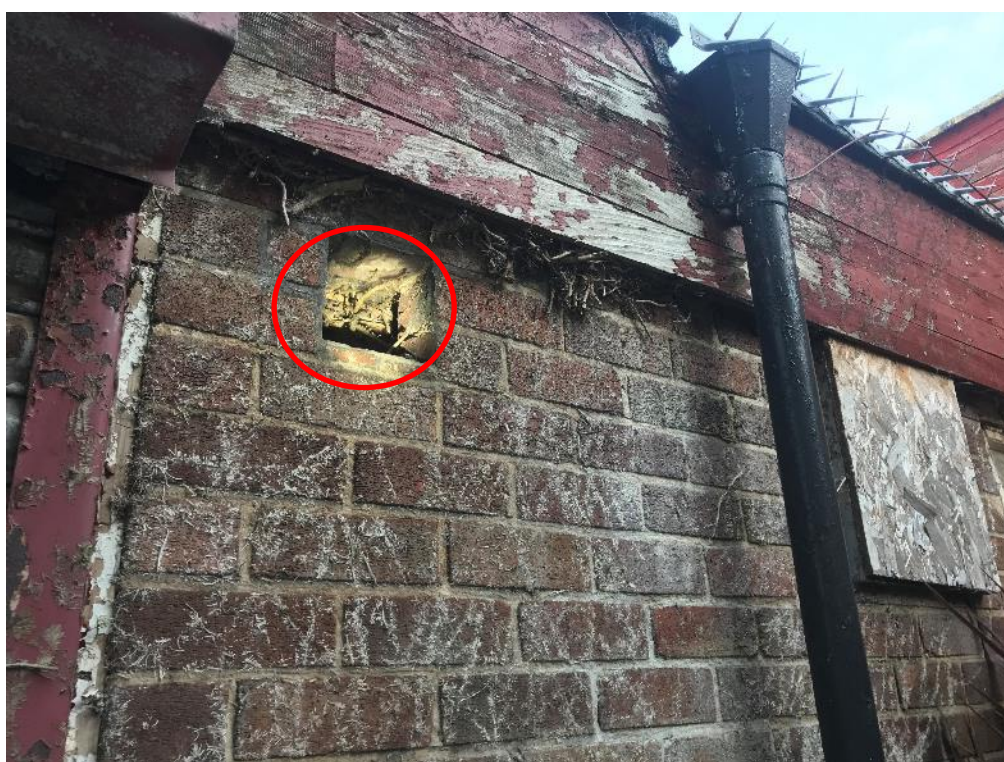
Plate 6 – Gap in the brickwork leading to the wall cavity on the south-eastern elevation
