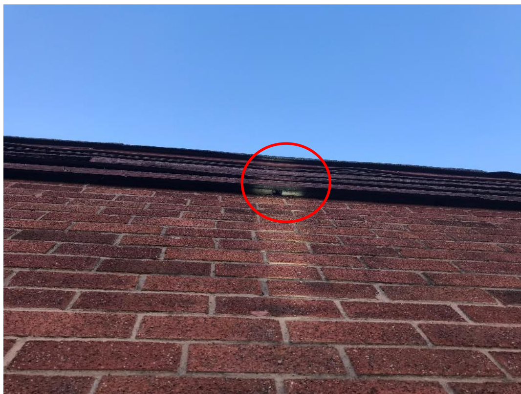
Plate 7 – Gap beneath the cladding on the western elevation
