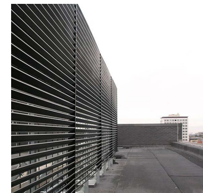
Louvred Screen at roof level
