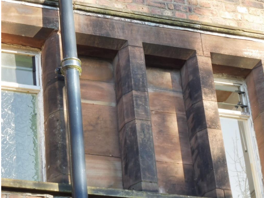
Photograph 17: Sample close up view of external stone work to village hall building. Note: The stone work is in good repair with no viable openings for bats or birds recorded.
