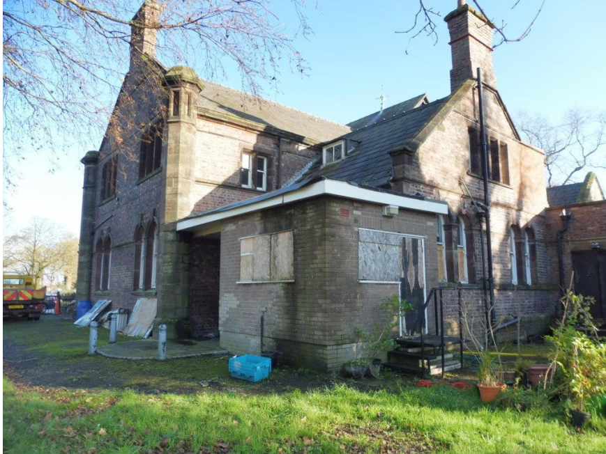
Photograph 5: View of west and south facing frontages to former Village Hall building..
