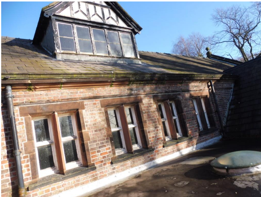
Photograph 6: Close up sample view of slate roofing on the Village Hall building.
