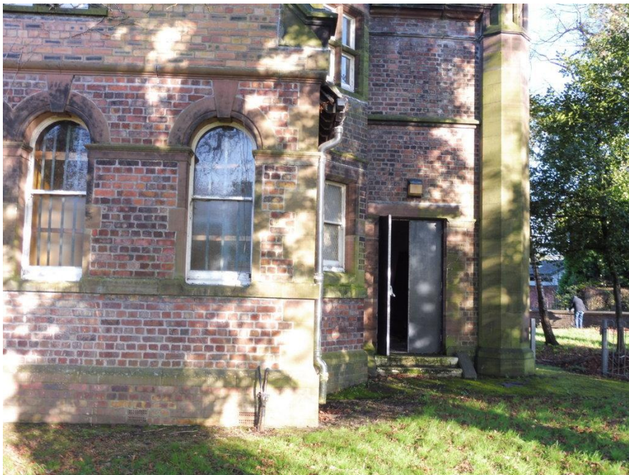
Photograph 18: Sample view of external brickwork to village hall building. Note: The brick work and mortar seal is in good repair throughout and well-sealed with no gapping or holes recorded through which bats could gain access.
