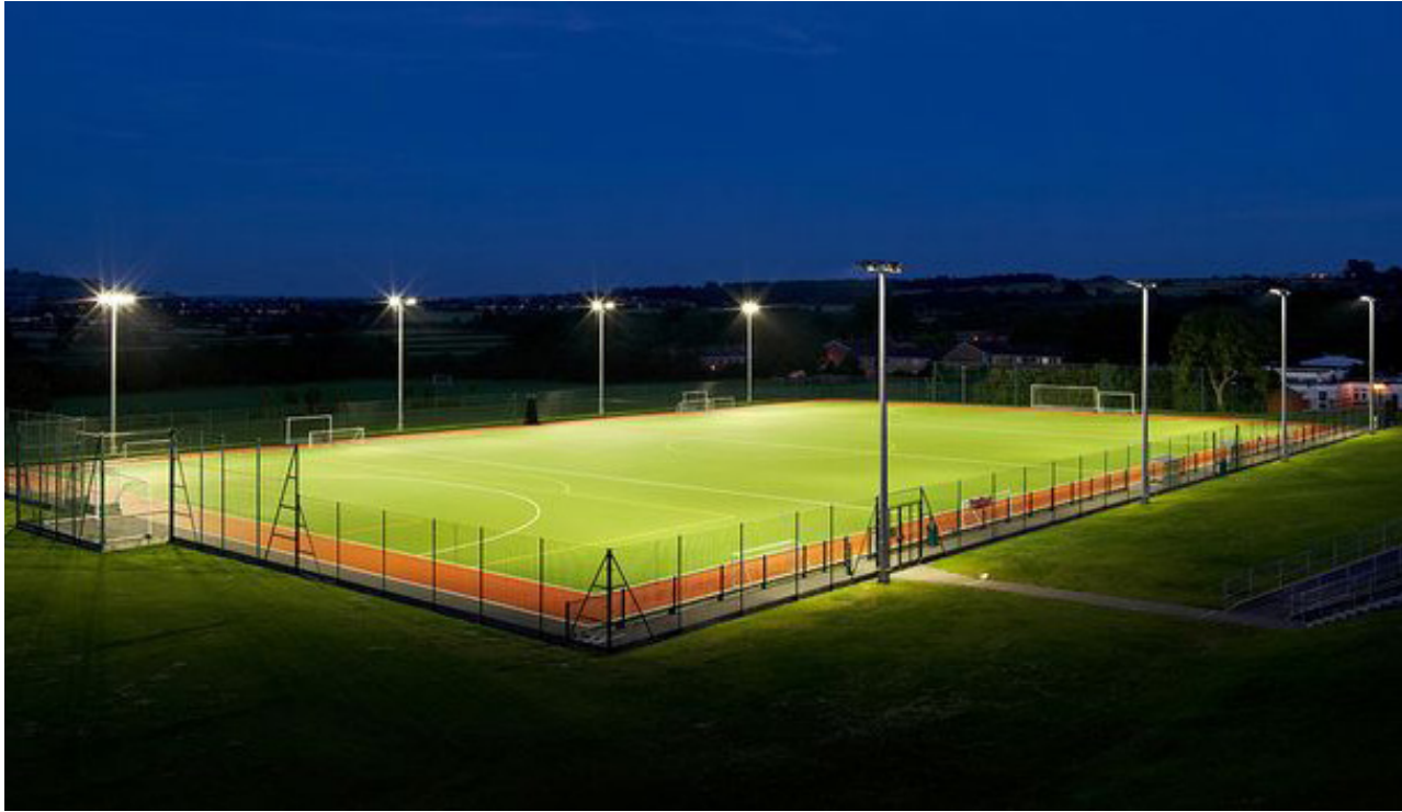
Column mounted floodlights
