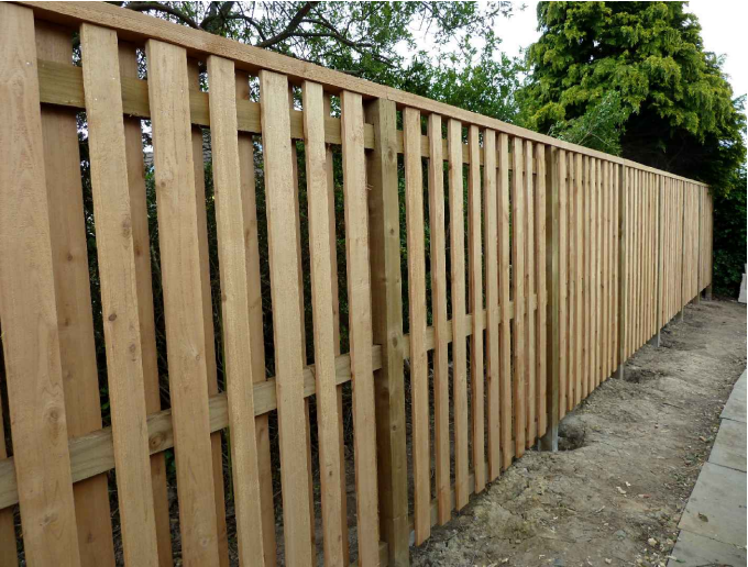
2.4m high Timber Hit & Miss Fence
