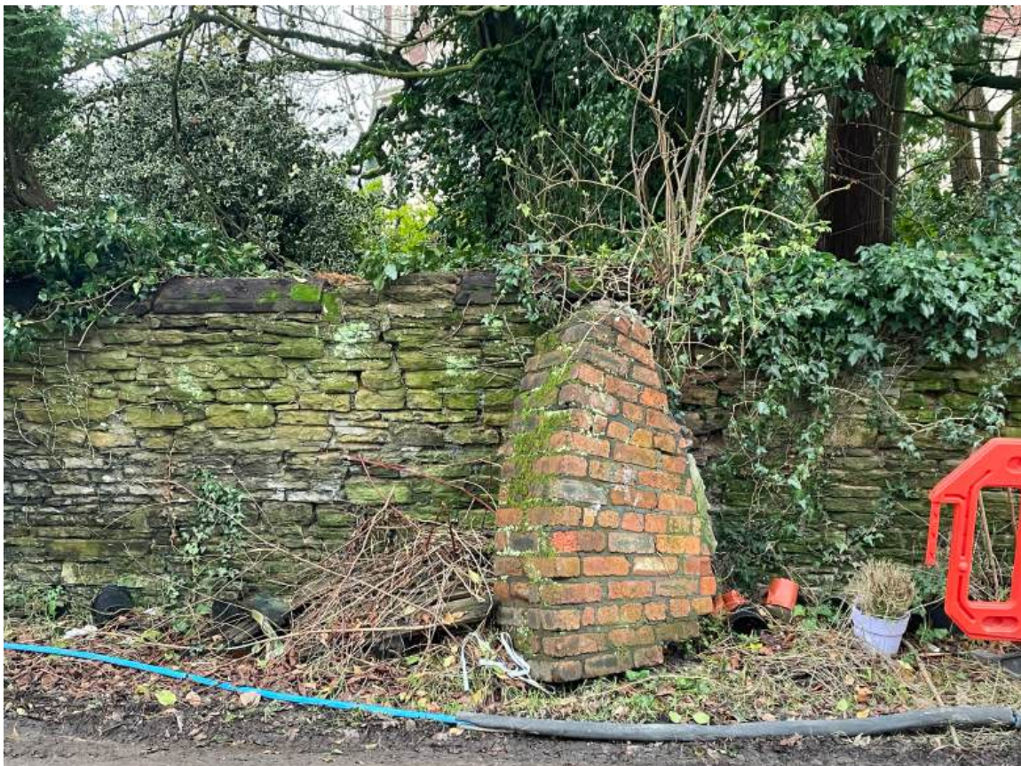
Photo 4: North Side of Wall - Broken Buttress
