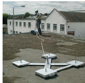
Temporary mansafe system (Level 06)
