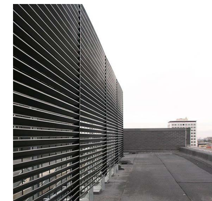
Louvred Screen at roof level
