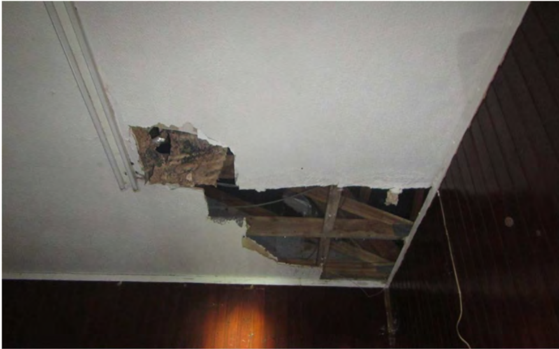
Photograph 21 – A damaged false ceiling within Building 7.
