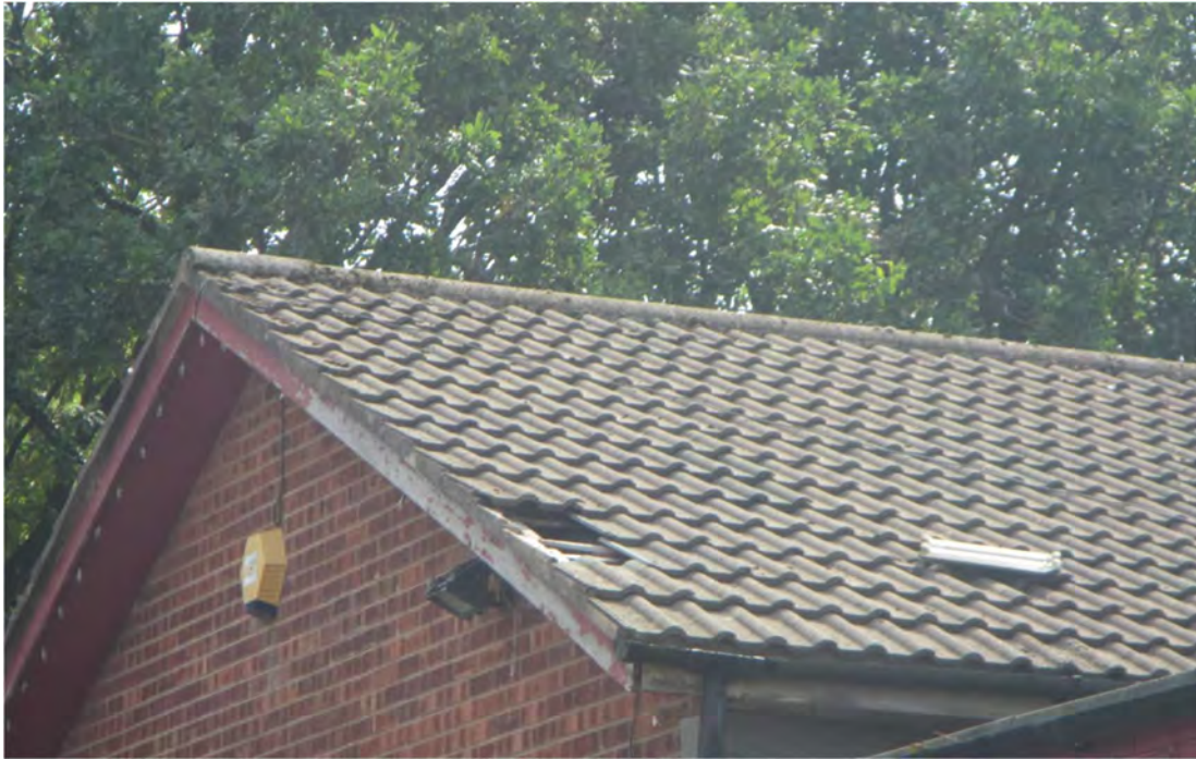
Photograph 17 – Missing tiles on the roof of Building 7.
