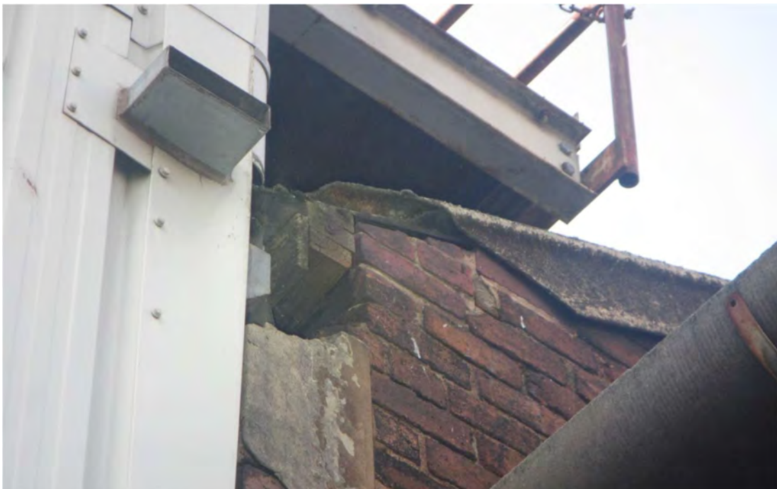
Photograph 8 – A gap between the top of the wall plate and the eaves of Building 1.
