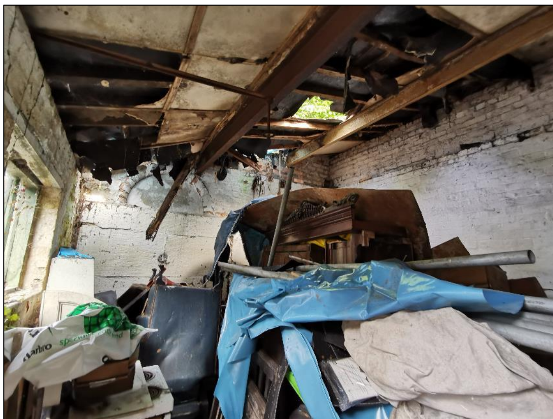
Plate 8 – Interior; western-most compartment, note hole in the roof
