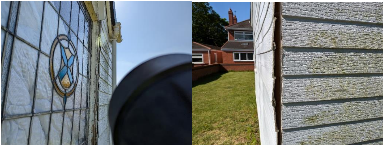
Plate 8 – B4 – low but potential value crevices in-behind timbers at corners and windows
