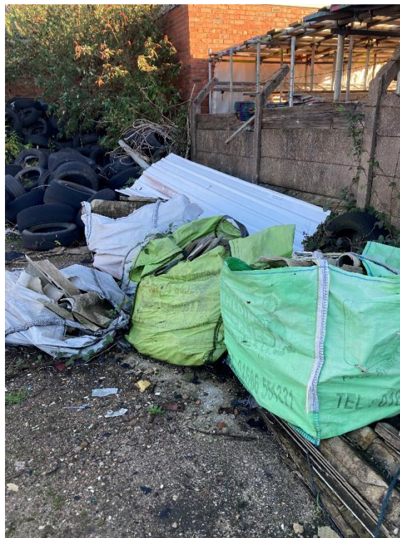
PLATE 2 BAGS CONTAINING ACM WASTE - NORTHEAST CORNER LOOKING NE
