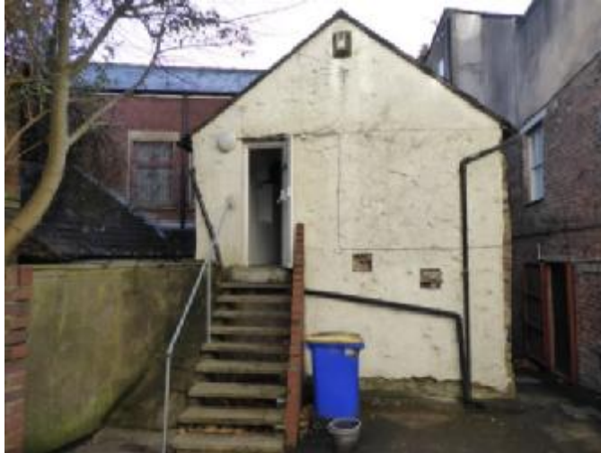
Rear Outrigger Gable with roughcast cement based render. (Image taken prior to the render removed as part of the works relating to planning application ref: 20/00724/FUL).
