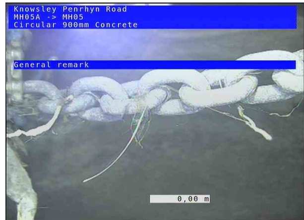
MH05A_b4263f91-a8fb-4f3c-9d3e-a8c5069213ef_20220427_143928_509.jpg, 00:00:17, 0.00 m General remark, CHAIN ACROSS THE OUTGOING PIPE IN MH05A
