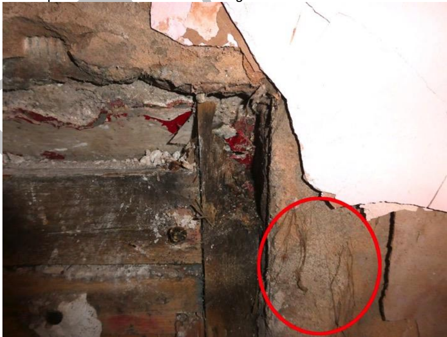
Figure 7. Mycelium growing on non-structural timbers and between plaster layers.
