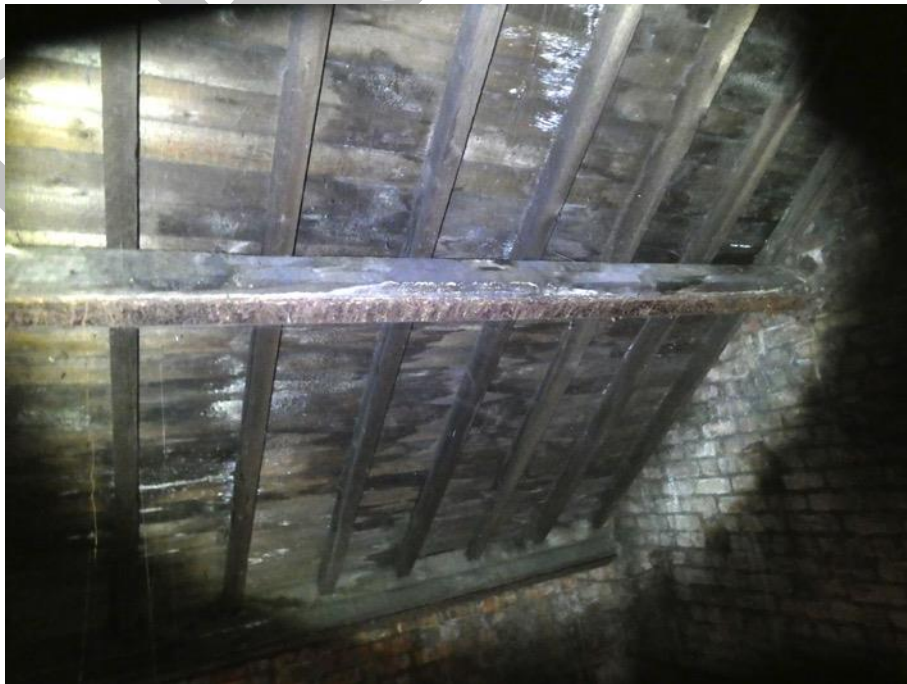
Figure 5. Fungal activity in purlin in south bay.
