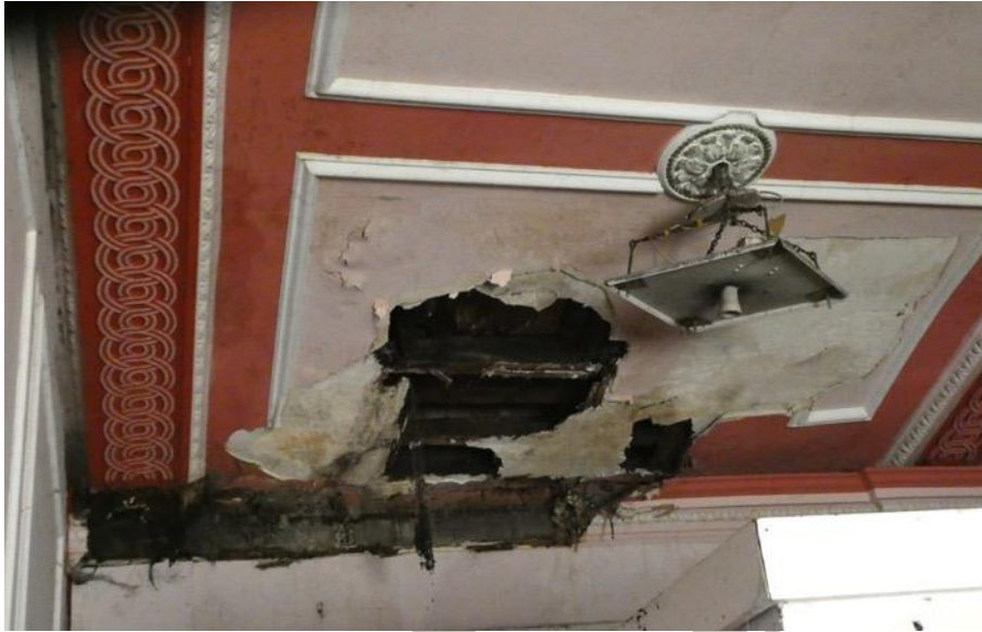
Figure 4. Damage to plaster ceiling caused by a roof failure directly above.
