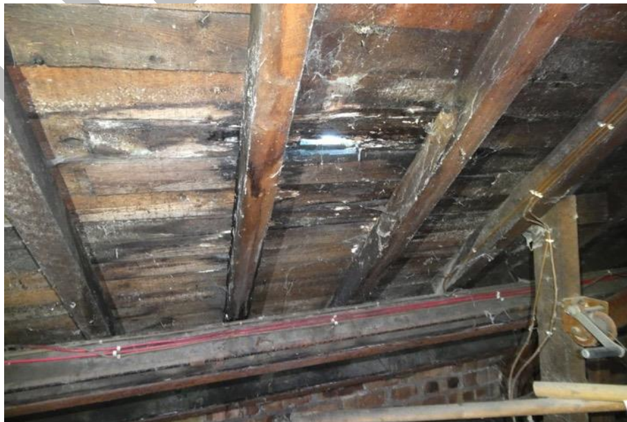
Figure 3. Localised decay of sarking boards.
