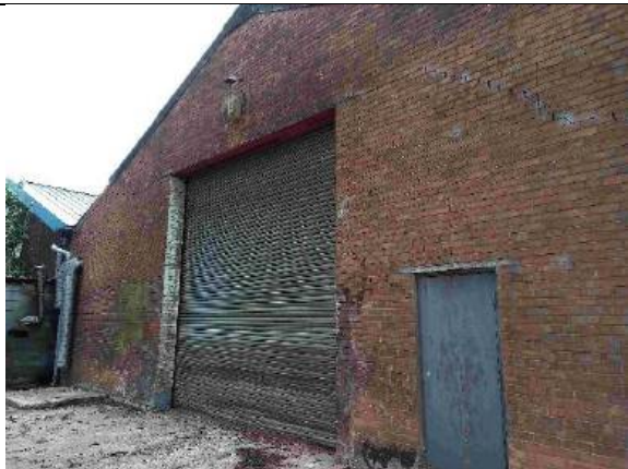
Photograph 15: Eastern elevation of B2 with large crack and missing pointing in brickwork
