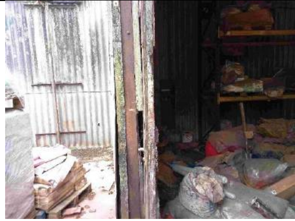
Photograph 12: Gaps between the sliding doors and wall on eastern elevation of B1
