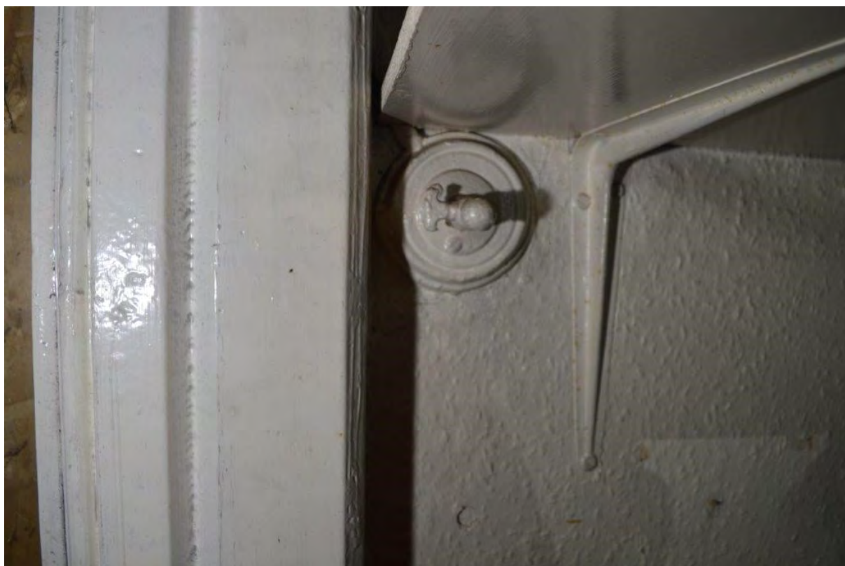
Plate 38. Light switch adjacent to window
