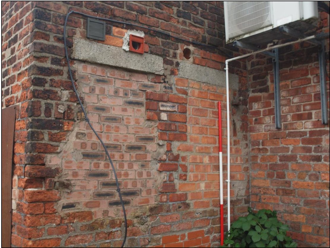
Plate 25: Detail of blocked windows
