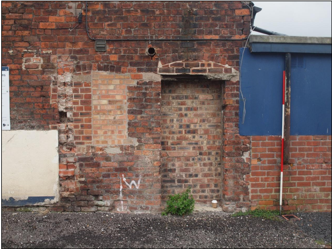
Plate 9: Blocked window and blocked doorway to lean-to extension
