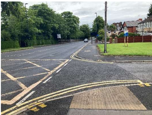
Photograph 5: Tactile Paving and footway conditions at the site frontage viewing eastbound along Huyton Lane
