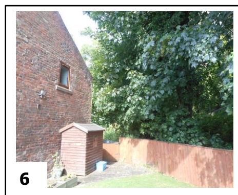
Photo 6: A view of the gable of the Coach House showing tree encroachment.
