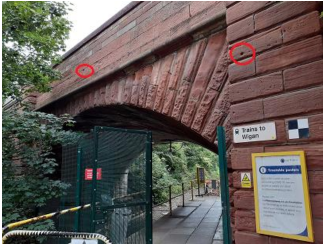
Photograph 15. Glovers Brow Bridge (eastern elevation) with crack to left and pockmark to right highlighted (red circles).
