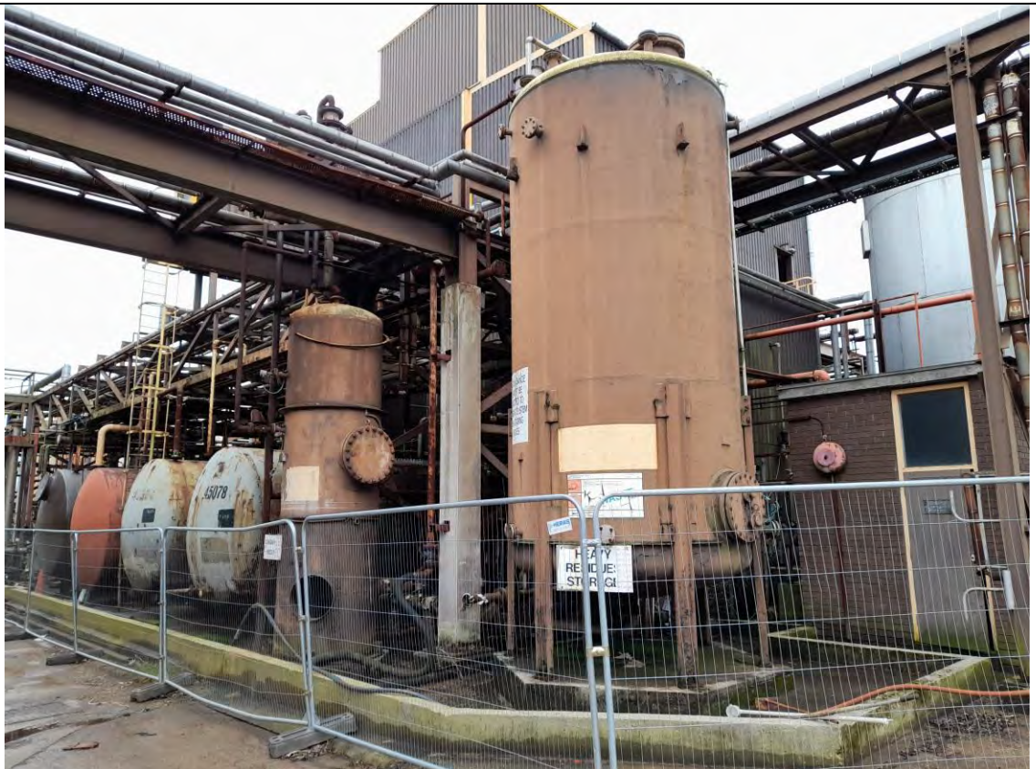
A17.4. View of the bundled tanks to the east of the Diol Plant
