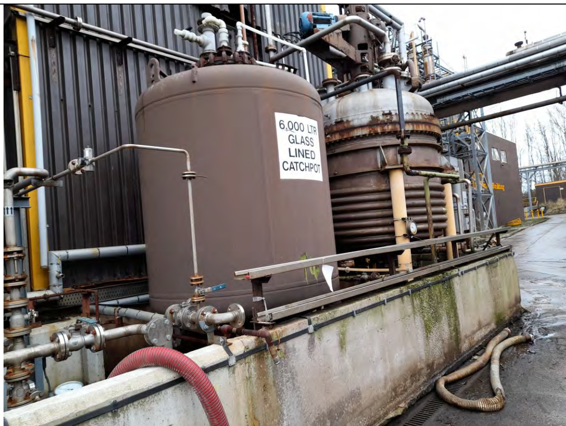
A15.3 View of the bunded tanks along the eastern side of the TDC building
