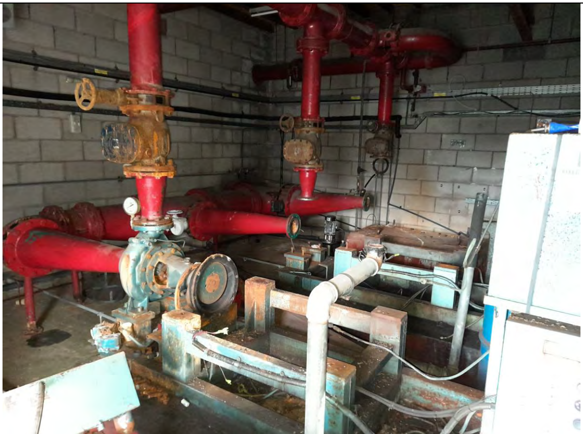
A1.2. Pipe work within the pump house
