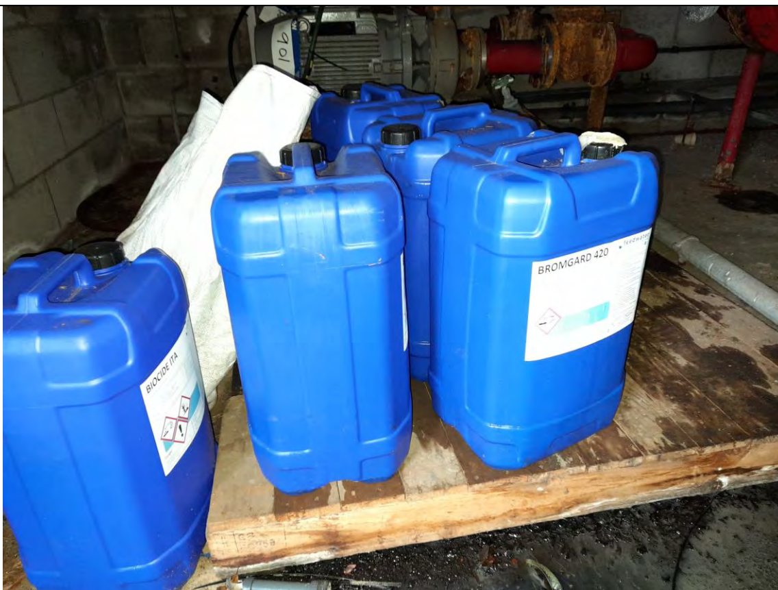
A1.3. Chemicals within the pump house
