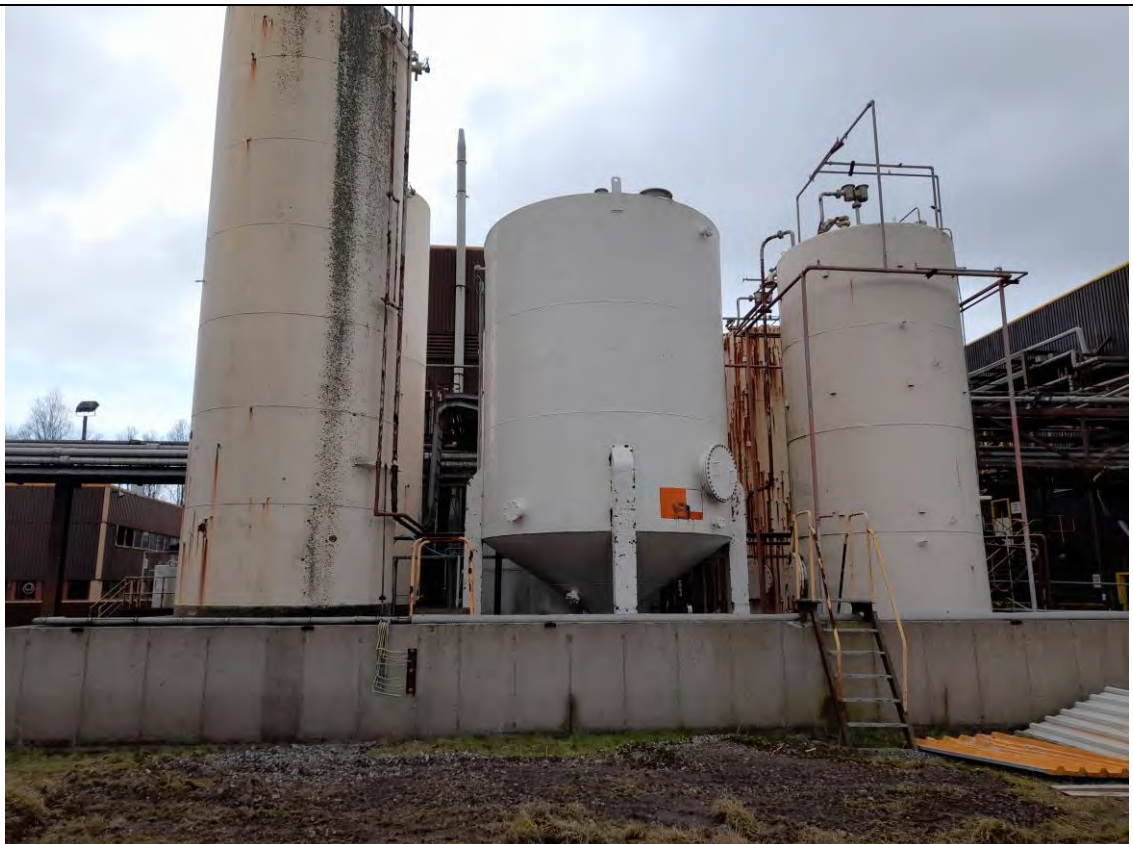
A17.2. View of the bunded tank farm to the south of the Diol Plant
