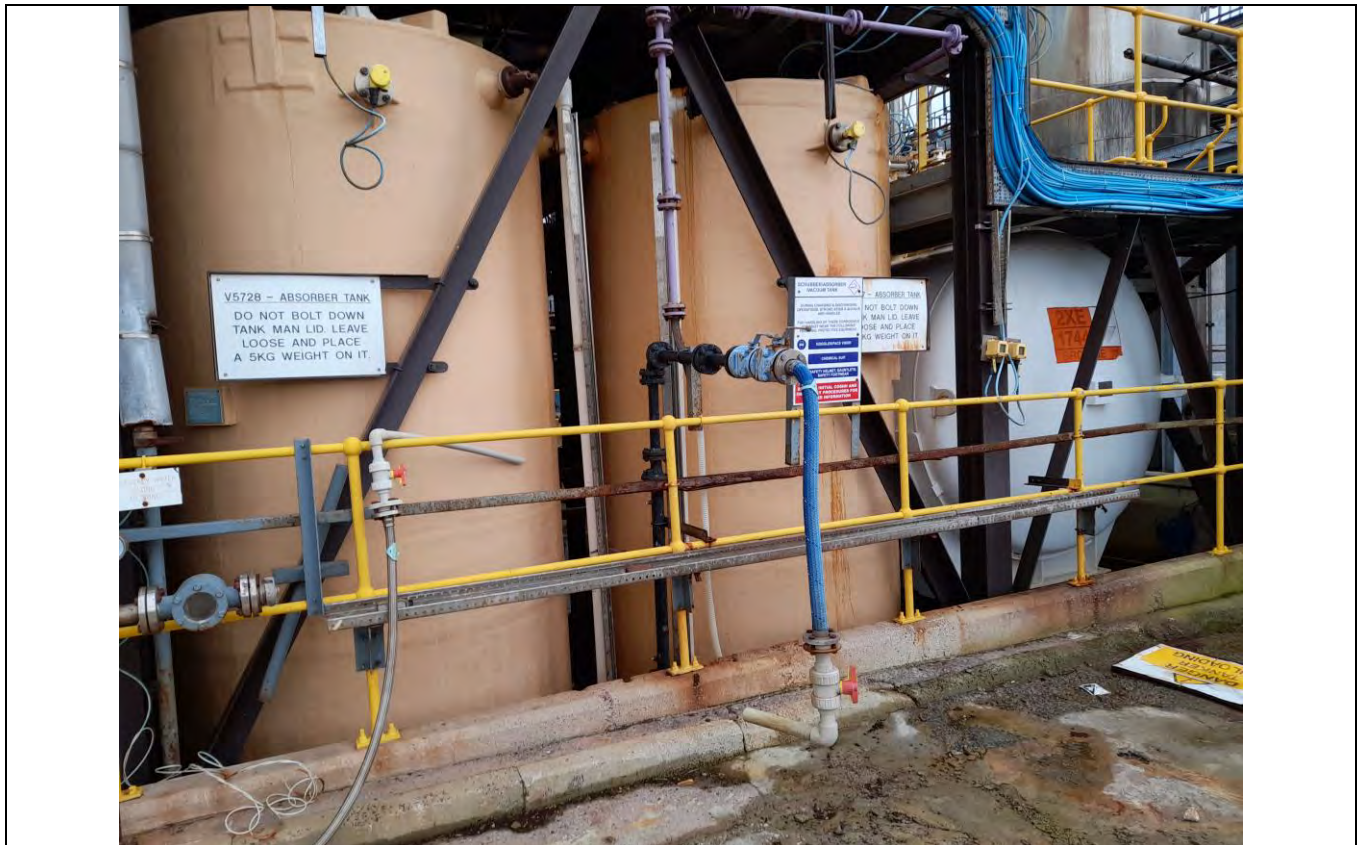
A16.3 View of the bunded tanks to the south of the Bonner building
