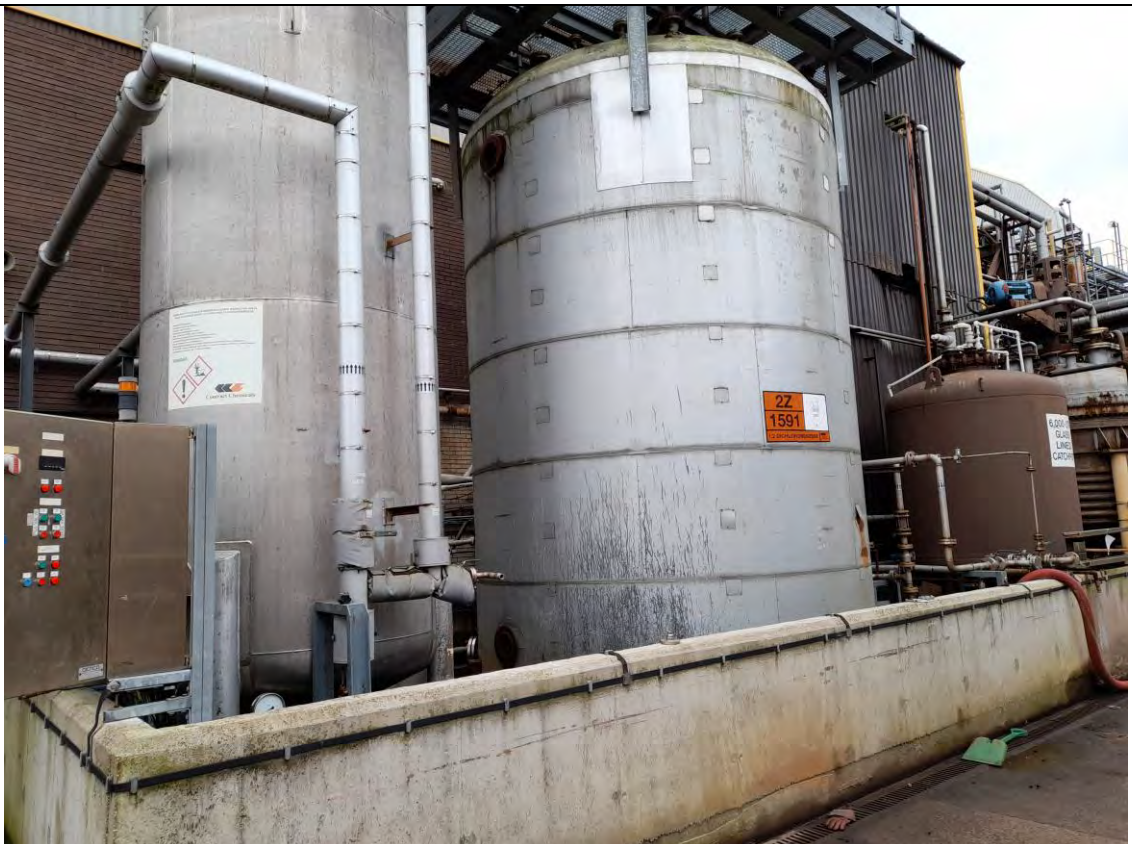
A15.2. View of the bunded tanks along the eastern side of the TDC building
