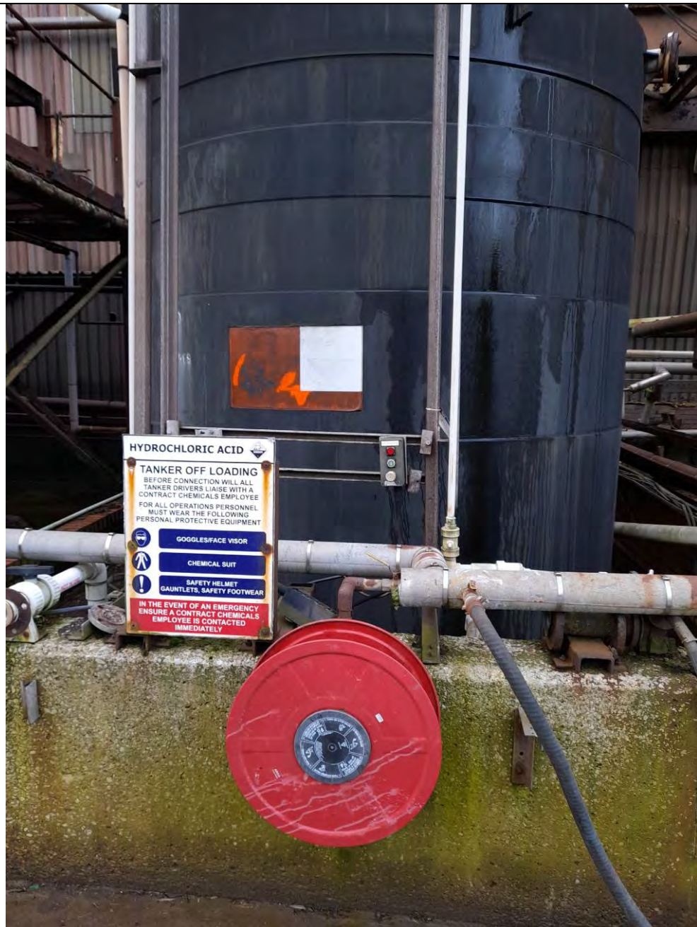
A5.5. View of tank in Surfactant tank farm
