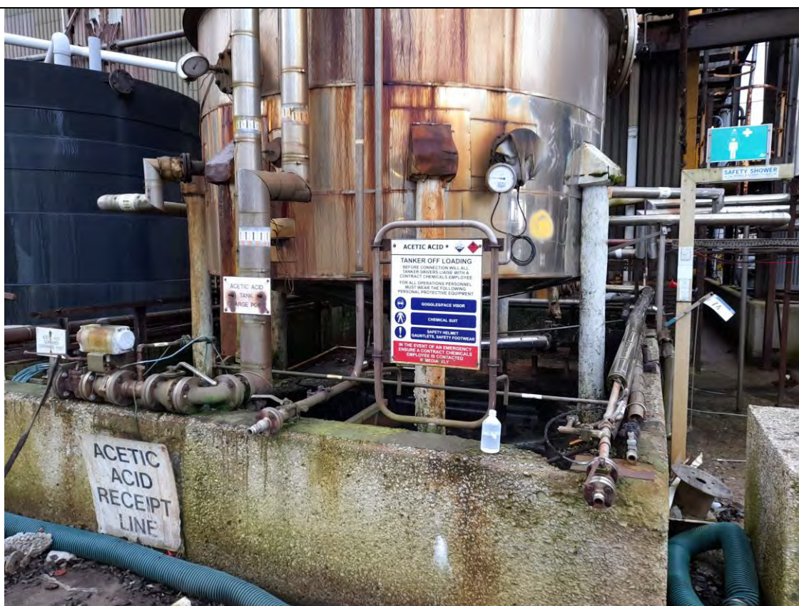
A5.4. View of tank in Surfactant tank farm
