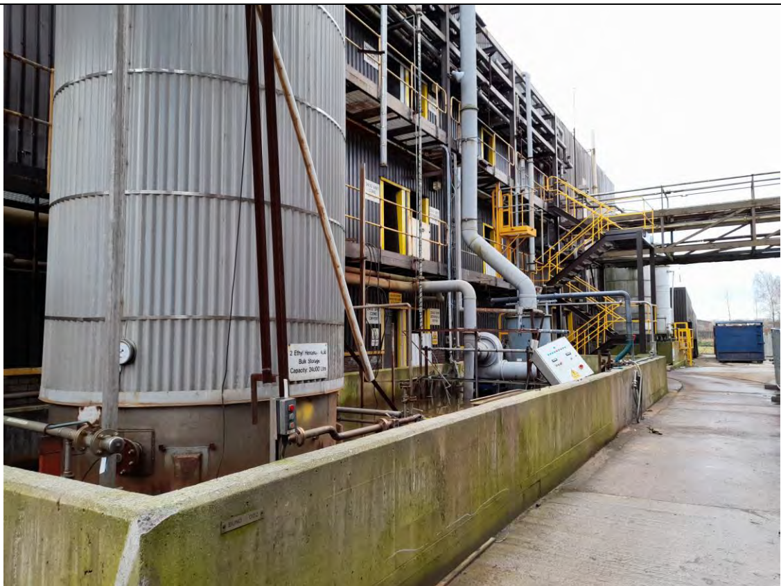
A5.2. View of the tank farm to the north of the Surfactant building
