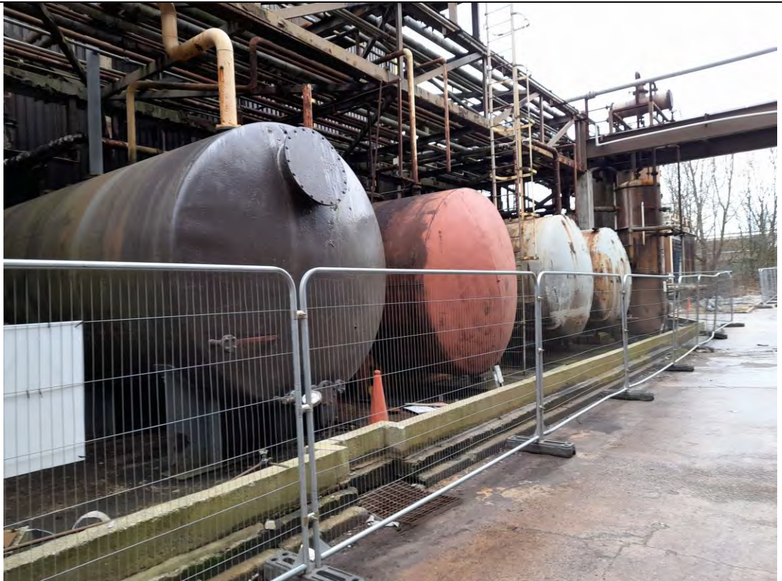
A17.3 View of the bundled tanks to the east of the Diol Plant
