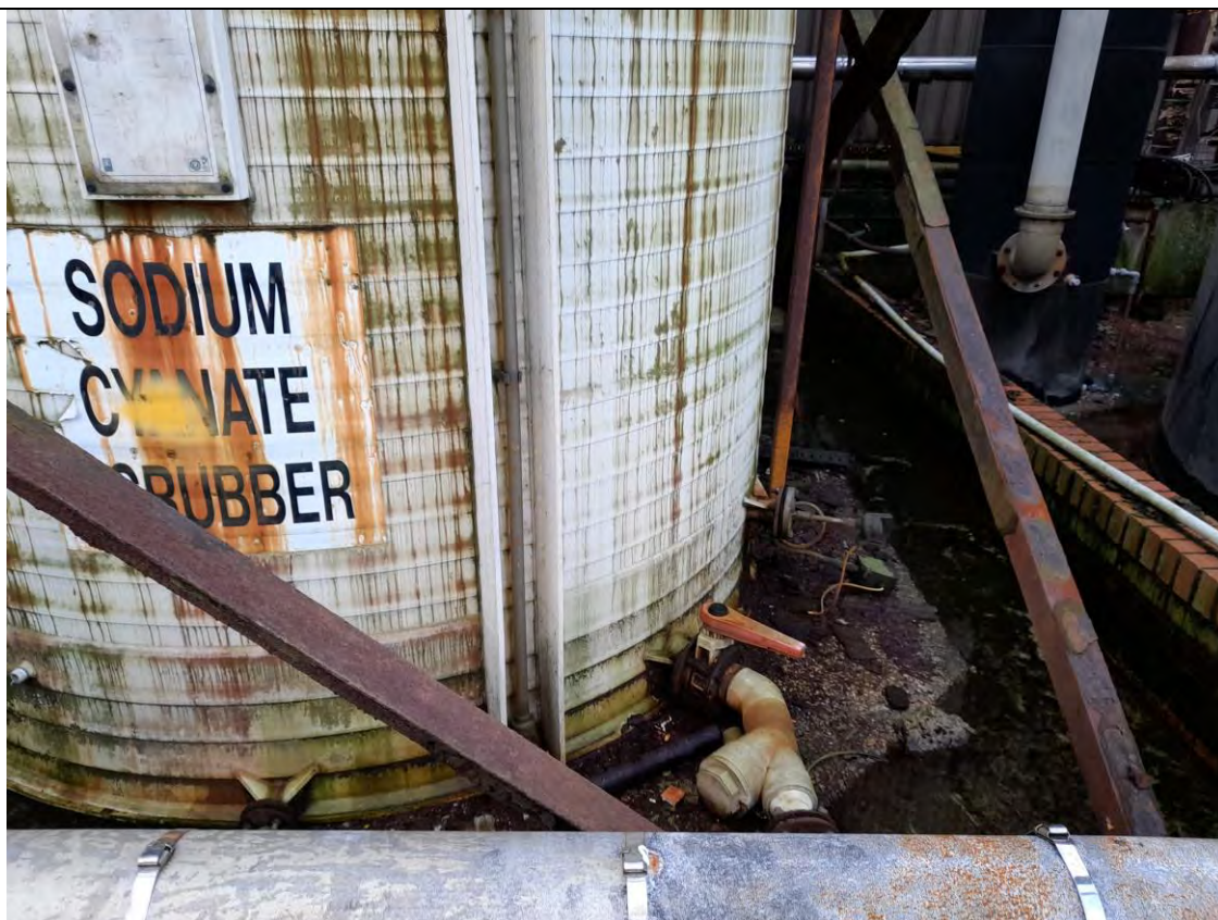
A5.3. View of tank in Surfactant tank farm
