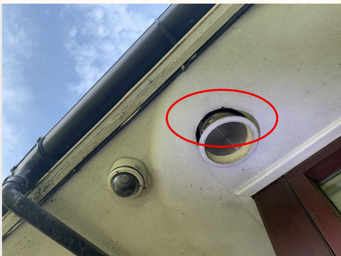
Photograph 5: Damaged light fixture with access into crevice, identified as a PRF.
