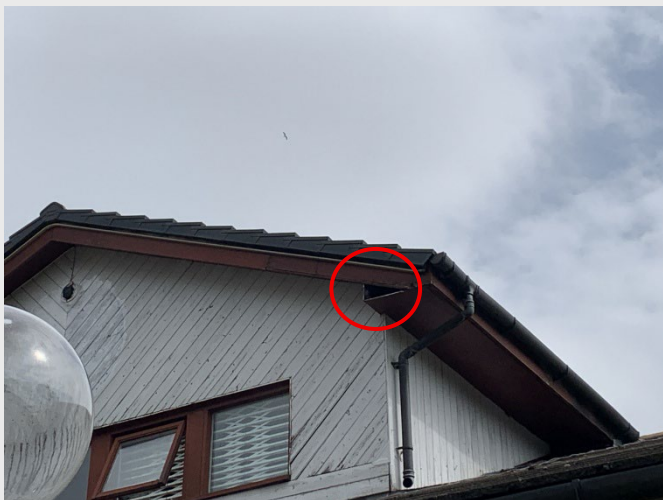
Photograph 7: Gap in roof gable verge, identified as a PRF
