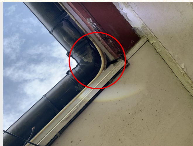
Photograph 6: Gap in-between soffit board of B1 with access into crevice, identified as a PRF.
