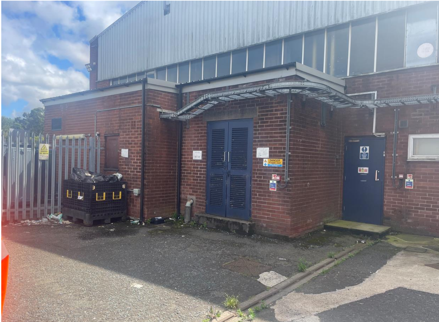
Photo 9: Gas inlet room with asbestos warning sites on building. Electricity substation is located in the left of photo.
