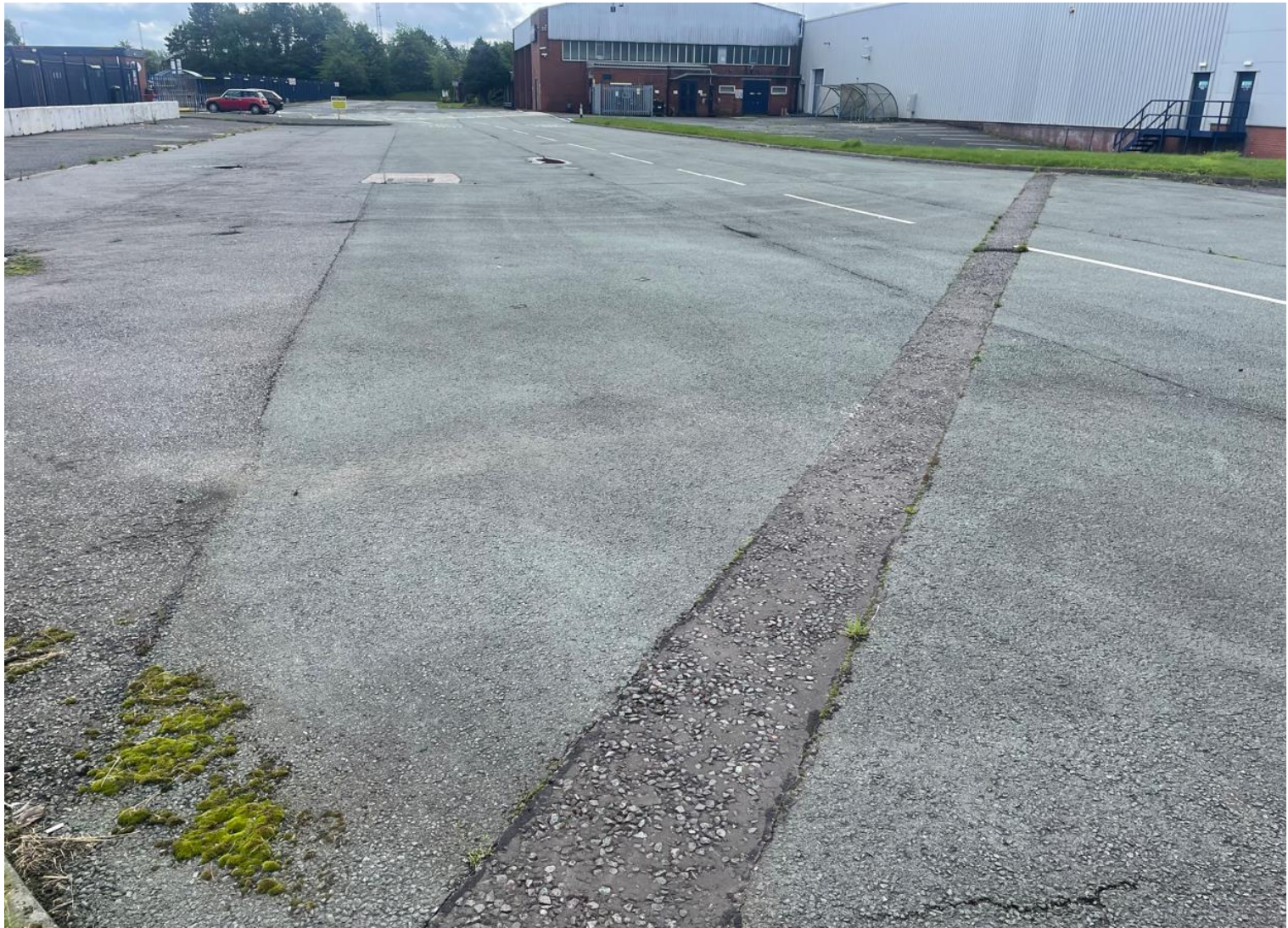
Photo 5: Possible buried services are indicated by scars in asphalt surfacing, located in north eastern parts of site.
