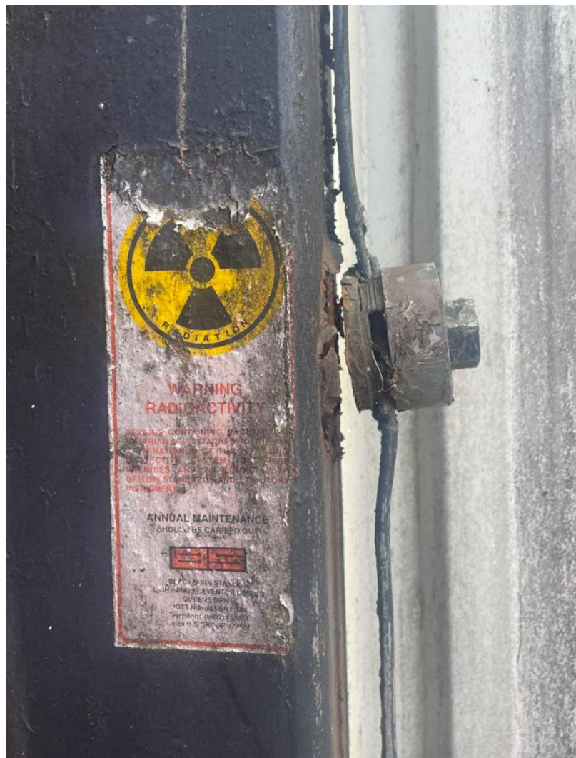
Photo 10: Dated radiation warning label on pole noted in Photo 8, likely electromagnetic. This may be associated with components of a former alarm system.
