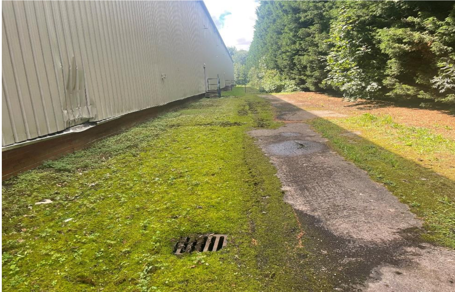
Photo 28: Tracking runs between the warehouse and northern site boundary (view is looking west). A surface drain and damage to the warehouse cladding is visible.
