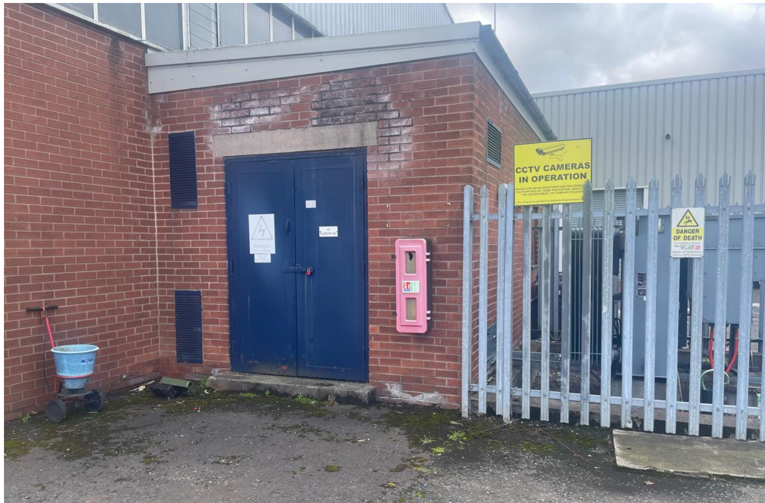
Photo 11: Electricity substation to the right of photo has warning signs of sulphur hexafluoride. LV building to the left of photo.
