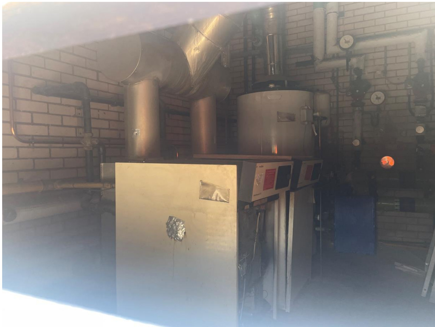
Photo 21: View into boiler house through broken section of door. Access into the boiler house was not granted, therefore a review of any potential tanks could not be undertaken.
