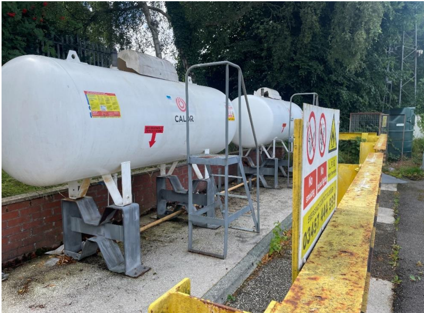
Photo 25: 2 No. Propane tanks (appear to be used for filling forklifts), located towards the southern site boundary.
