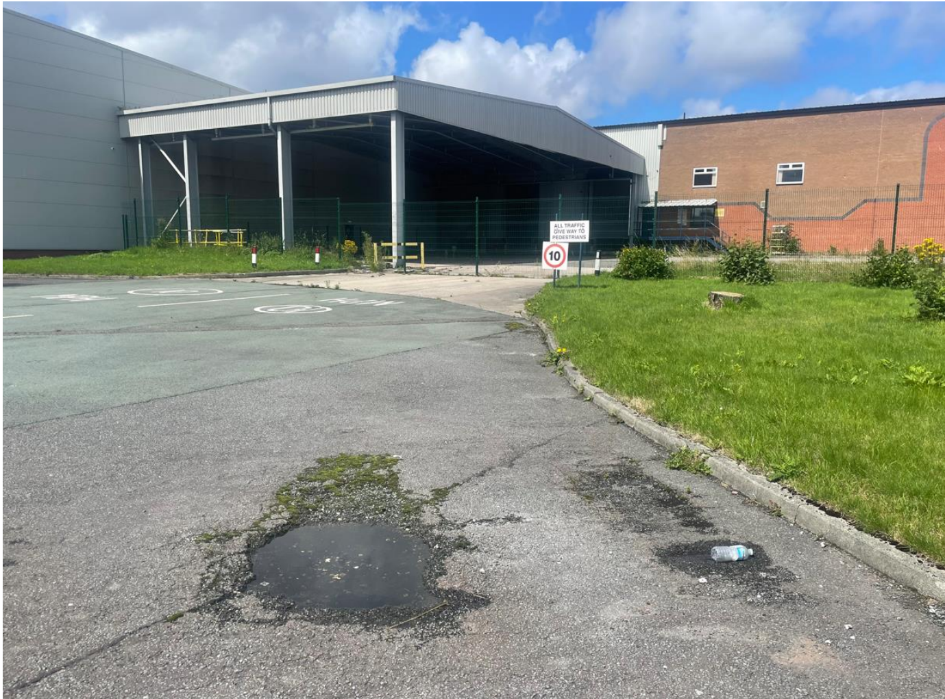
Photo 1: View looking north fo localised deterioration of hard surfacing on access road in north eastern part of site. The buildings beyond the palisade fencing are offsite. Soft landscaping areas partially border the northern site boundary on the eastern side.
