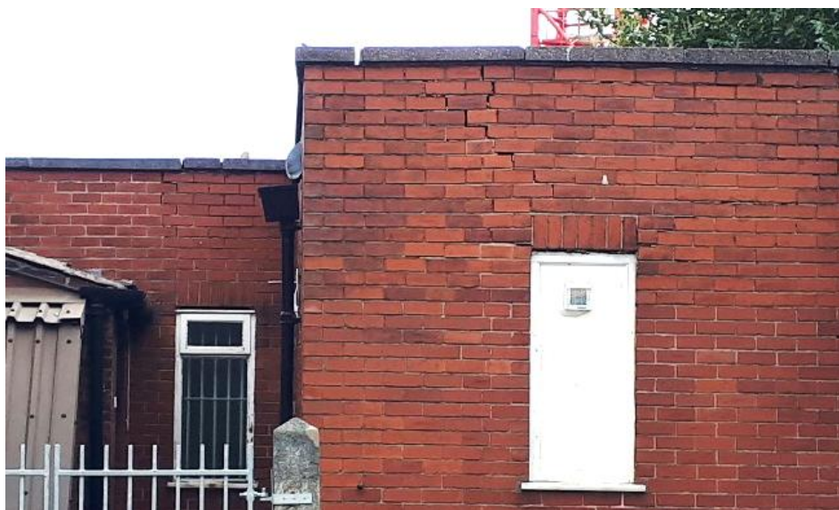
Figure 8: Typical instance of cracking and open perpendicular joints in one-storey extensions to the south.
