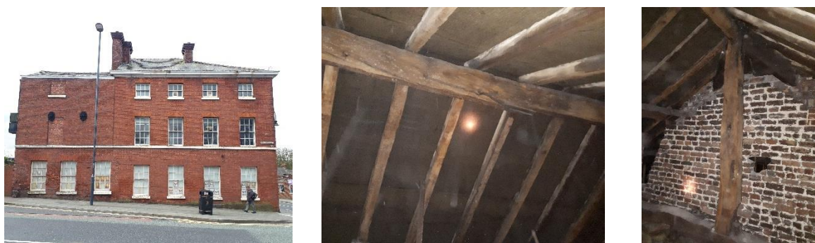
Figure 2: Sagging ridgelines (left), structural defect on ridge purlin (centre), and prop supporting hipped roof connection (right)
