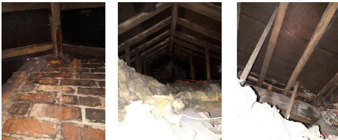
Figure 3: Ridgeboard at bearing on main gable chimney with water ingress (left), view of ridgeboard and arching common rafters (centre), and areas of damp on south roof slope (right).
