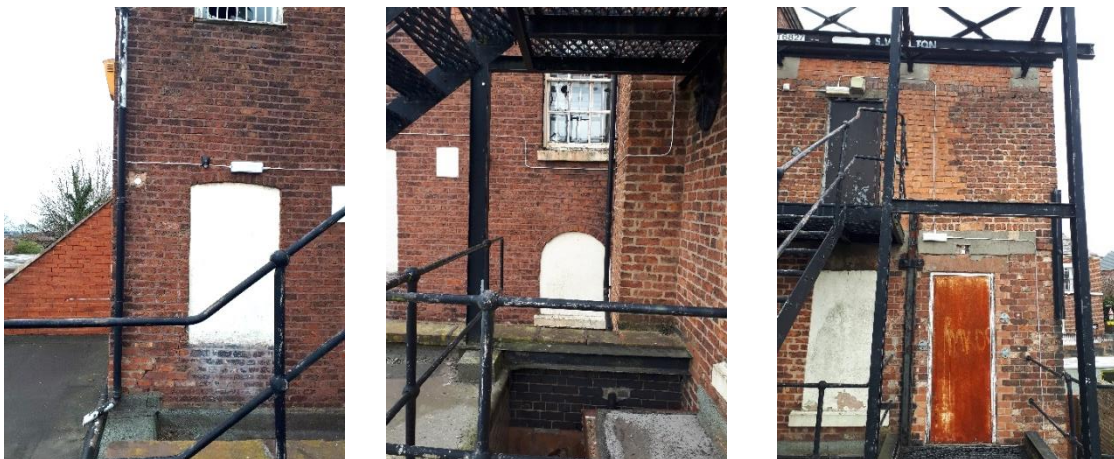
Figure 7: Cranked bed-joints at interface with main gable (left and centre), and steel lifting structure with larger opening that has not been properly made good (right).
