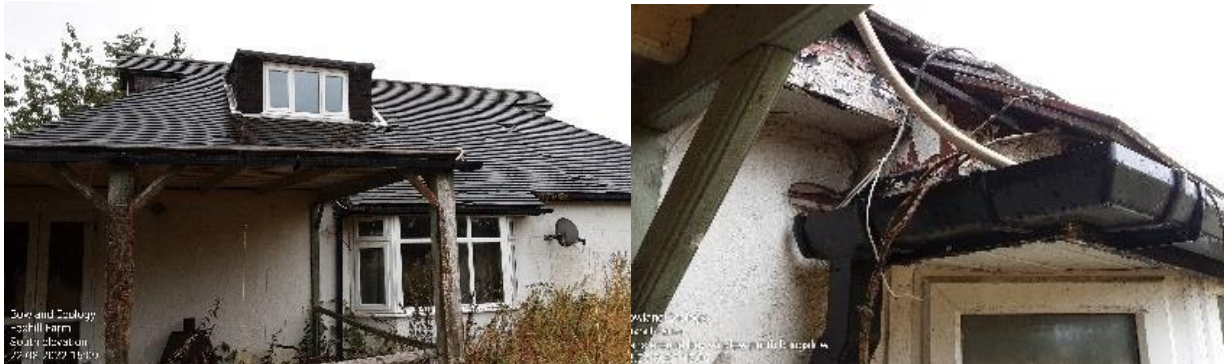
Plates 21 and 22: Dormer on south-western elevation and gaps at adjacent bay window
