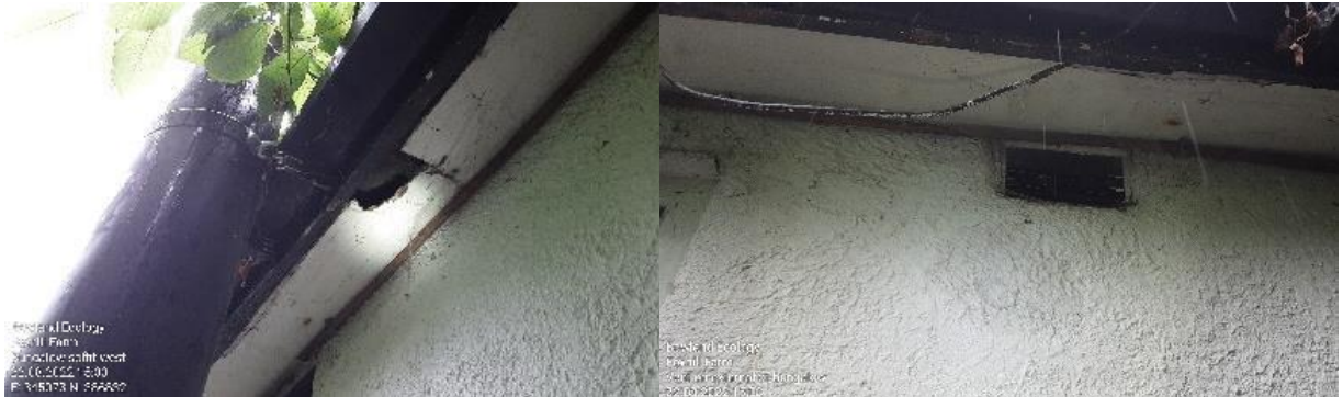
Plate 23 and 24: Eastern elevation hole in soffit box and air vent
