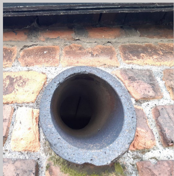
Photograph 16: Piggery ventilation tubes
