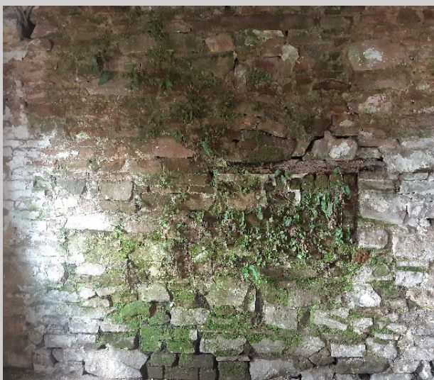
Photograph 11: Stone Barn A – B adjoining wall damage
