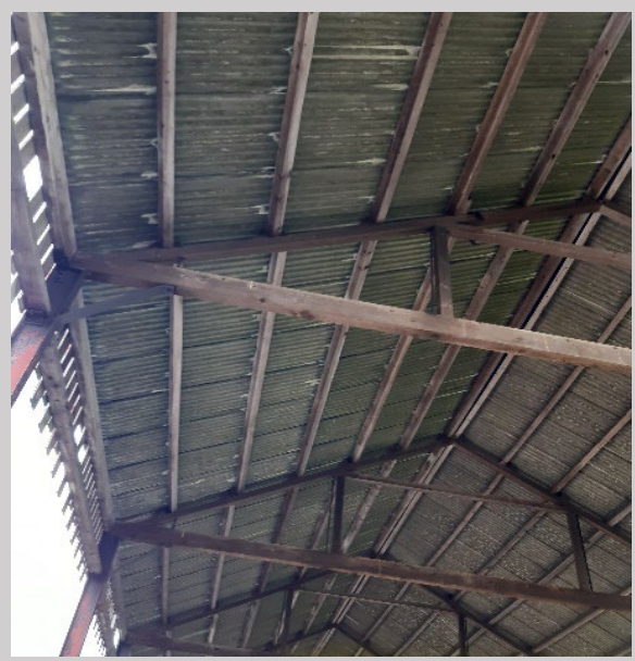
Photograph 14: Main Barn unlined roof
