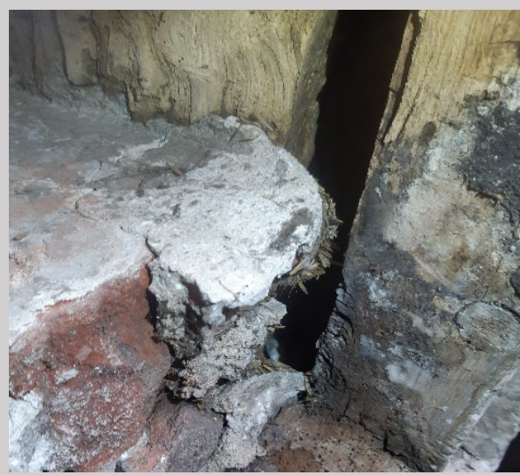
Photograph 12: Stone Barn B window frame cavity
