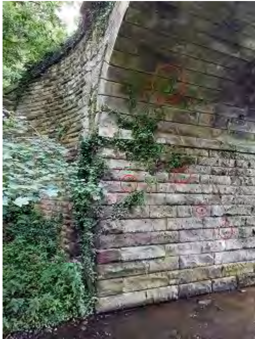
Photograph 21. Cracks and pockmarks in Millbrook Bridge over stream.
