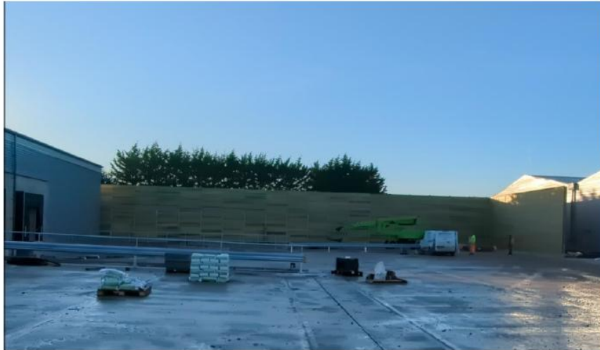
Unit F acoustic fence
