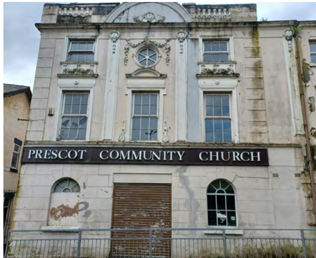
Note the vertical crack on the parapet and at ground floor. This is possibly the original building line with everything to left the mid-late 19th century extension.
