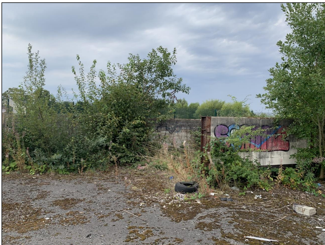
Plate 14 – Extant walls of a demolished / collapsed structure
