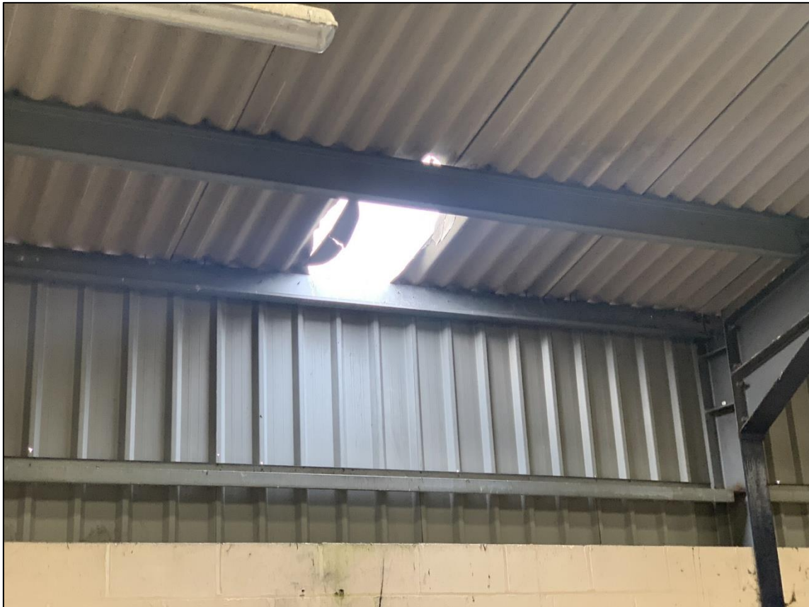
Plate 5 – Open hole in roof
