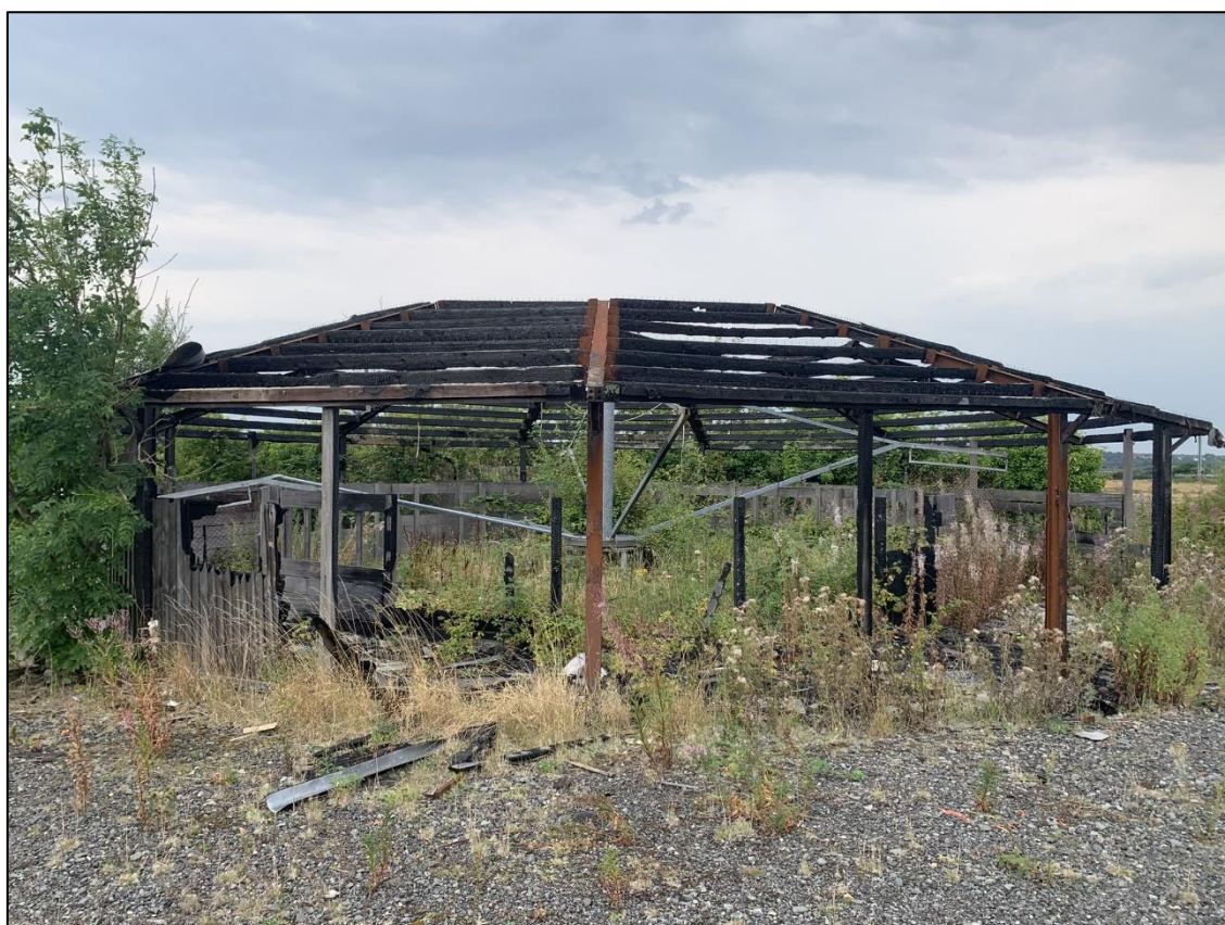
Plate 8 – Building B2, clearly burnt out
