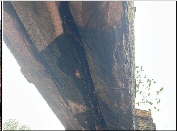
Figure 26: Gaps between lintels.
