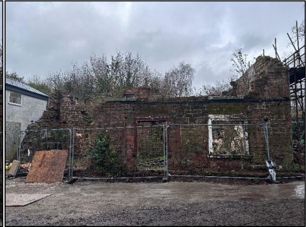
Figure 14: The ruined building.
