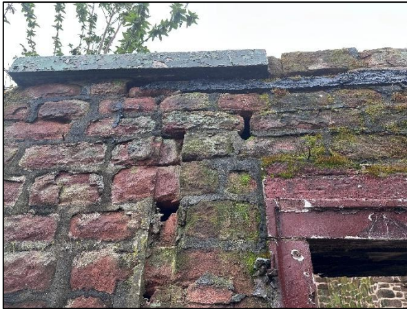
Figure 25: Voids in the walls of the building.
