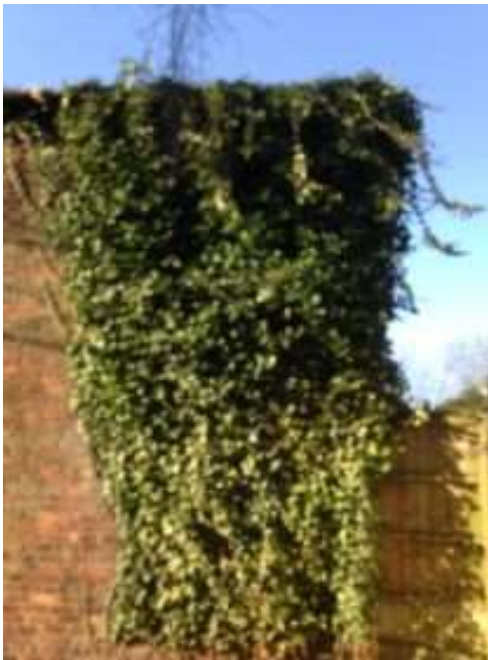
Plate 2 – Vegetation growth to the east end of the south frontage of the stable block.
