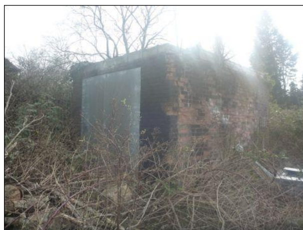
Photo 72: Structure 4, a fire damaged metal boarded brick structure
