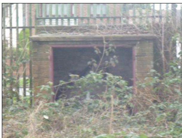
Photo 71: Structure 3, an open fronted and dilapidated outbuilding
