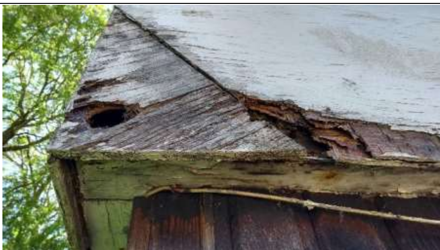
Photo 6: Holes in wooden fascias near the eastern corner of Building 2.
