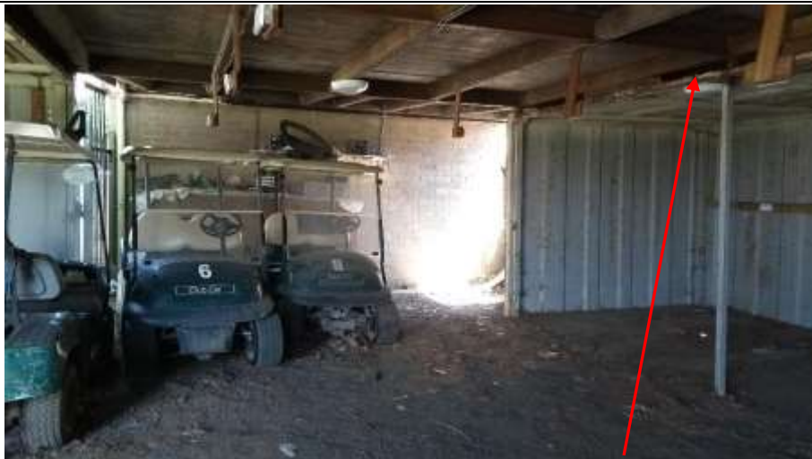
Photo 11: Internal area of Building 4. Arrow showing cavity between roof and shipping container.
