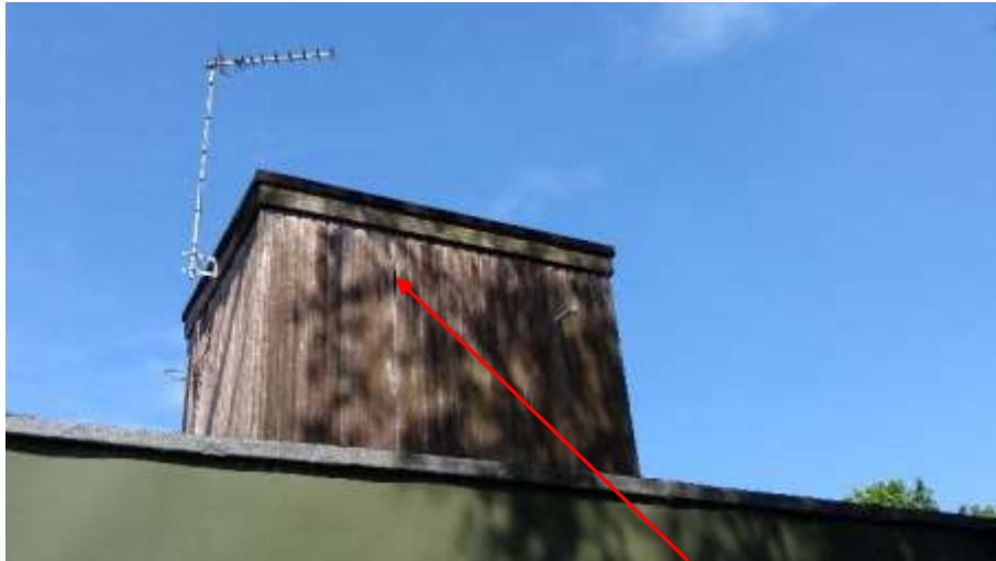
Photo 2: Centrally located wooden-clad stairwell shelter on Building 1. Arrow shows gap in cladding on the south-western elevation.
