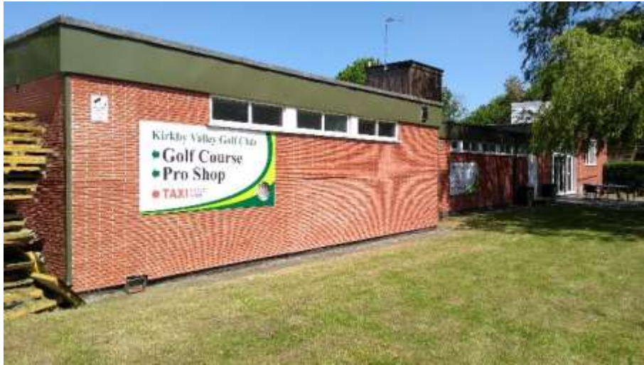
Photo 1: South-western elevation of Building 1. Where there are gap between cladding.
