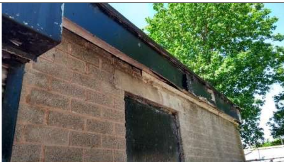
Photo 8: Showing poor condition of fascias on Building 3.
