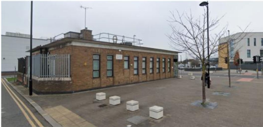
Showing jet cowl on the roof
