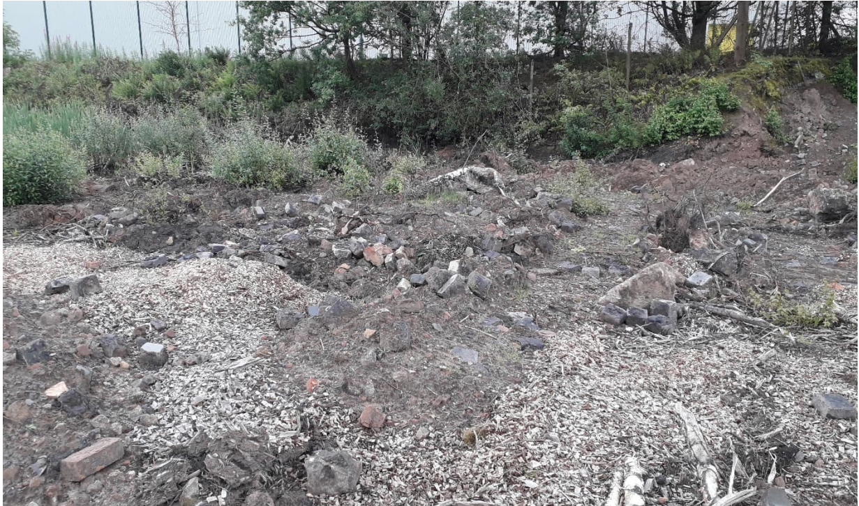
Figure 3-2: Areas of rubble within the site, looking west (WSP, 2020)
